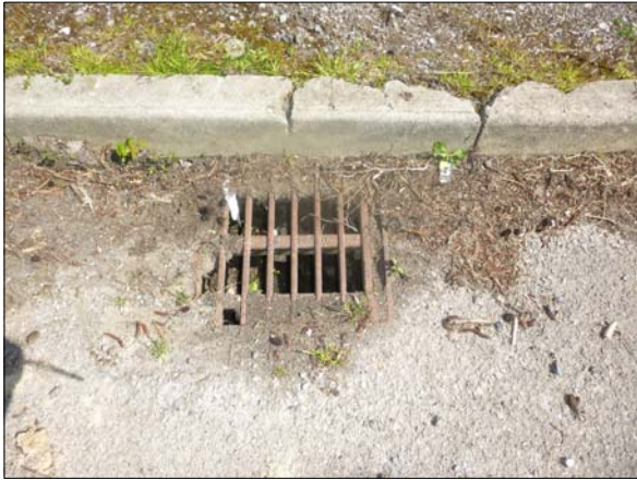
Title: GP31 Date: 14/5/18 Description: YARD GULLY No.2
