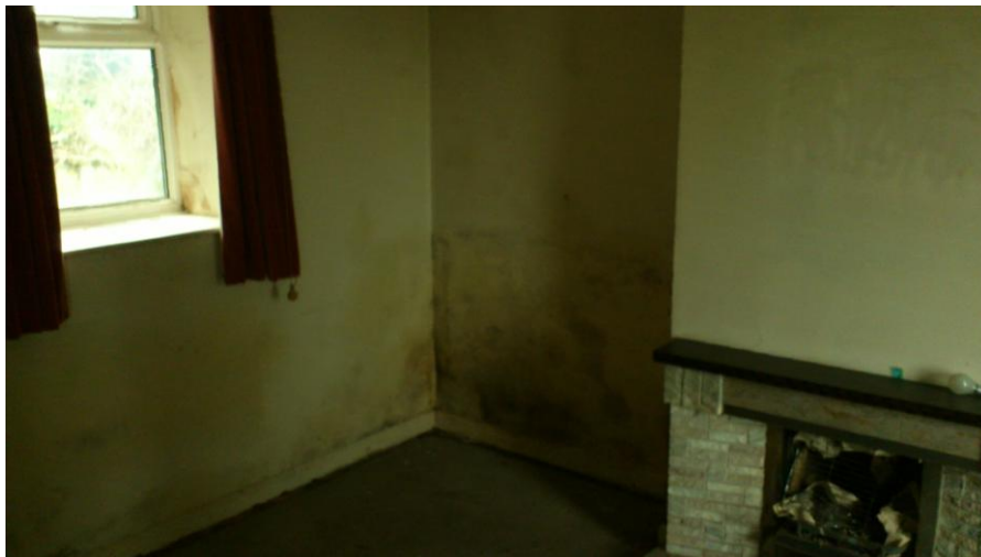
Sitting room with fire place and dampness to rear wall
