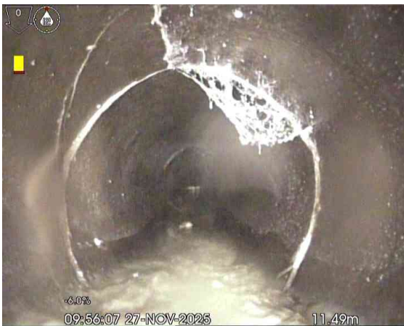
MH2X_3bcb78c7-9466-4ae2-86ac-98095ff7e9eb_20260313_111527_995.jpg, 00:04:30, 11.49 m Fracture, circumferential from 7 o'clock to 5 o'clock
