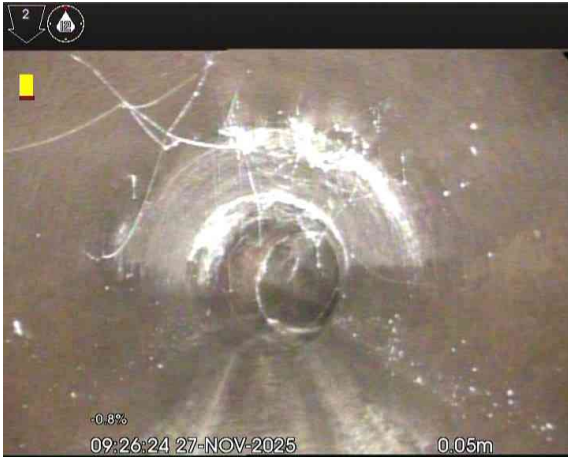
MH1X_1ef76ac6-41e7-4ec6-aeab-63b885e3d126_20260313_110729_063.jpg, 00:00:07, 0.05 m Attached deposits, grease from 5 o'clock to 7 o'clock, 5% cross-sectional area loss, start
