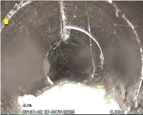
MH2X_818ccc4f-4d18-4b40-a918-19a349e1c481_20260313_111212_214.jpg, 00:00:12, 0.88 m Attached deposits, grease from 4 o'clock to 8 o'clock, 10% cross-sectional area loss
