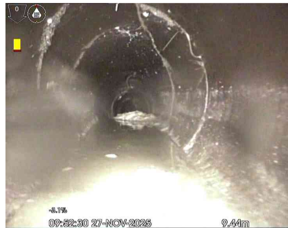
MH2X_0a784509-5fd1-46b5-a05f-f4a0b1826d82_20260313_11325_191.jpg, 00:00:54, 9.44 m Fracture, circumferential from 1 o'clock to 10 o'clock
