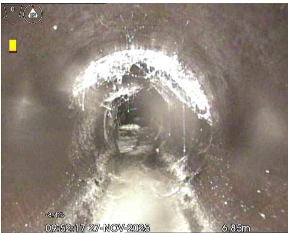
MH2X_2cd86d5a-0bc1-4e9f-bfdd-121cd456e43b_20260313_111249_014.jpg, 00:00:40, 6.85 m Roots, mass at joint, 10% cross-sectional area loss
