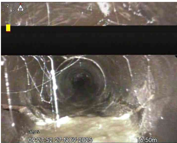
MH1X_c5e72bca-ab1e-47e4-b2b0-fdf1b0bdf871_20260313_10916_248.jpg, 00:01:35, 16.50 m Attached deposits, grease from 4 o'clock to 8 o'clock, 10% cross-sectional area loss
