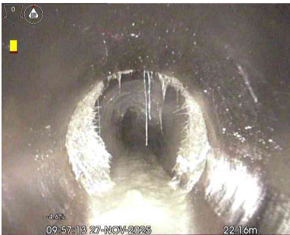
MH2X_a76a320c-37f5-43eb-9a43-85023a281dd6_20260313_112453_809.jpg, 00:05:36, 22.16 m Roots, mass at joint, 30% cross-sectional area loss
