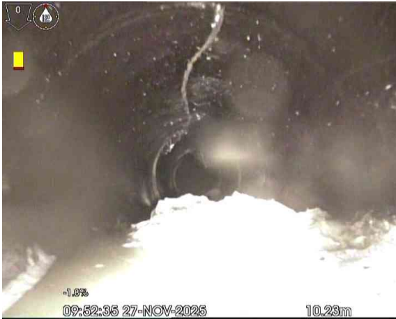
MH2X_2427d6f1-13ad-4109-b593-68367503c7bf_20260313_111343_072.jpg, 00:00:58, 10.23 m Attached deposits, fouling from 4 o'clock to 8 o'clock, 30% cross-sectional area loss
