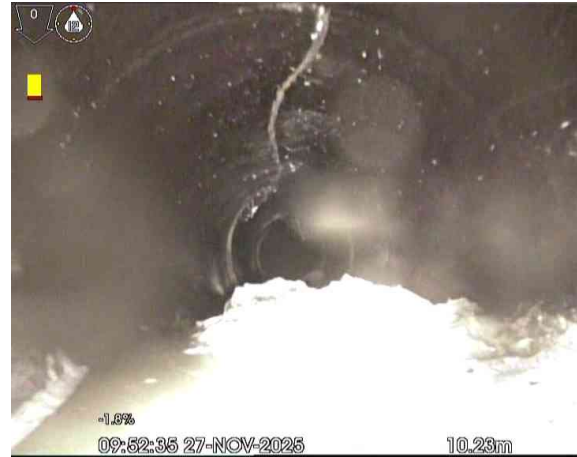
MH2X_b1274143-8e96-4b84-9351-5c0bf6a2b666_20260313_111354_664.jpg, 00:00:58, 10.23 m Fracture, longitudinal at 11 o'clock
