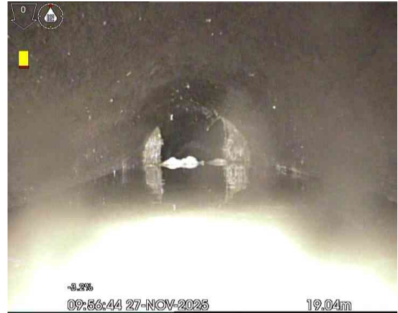
MH2X_d9ce8218-a954-494d-88f3-7a2f89db1e44_20260313_112415_637.jpg, 00:05:08, 19.04 m Roots, mass at joint, 30% cross-sectional area loss
