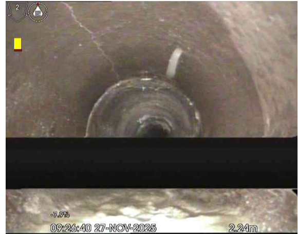
MH1X_52e127da-3993-4244-b0b5-3e04b4c125a6_20260313_110819_280.jpg, 00:00:23, 2.24 m Attached deposits, grease from 4 o'clock to 8 o'clock, 10% cross-sectional area loss
