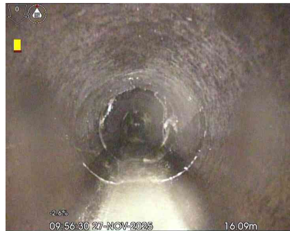
MH2X_192a24cd-58bd-432e-b754-3e98566dda8c_20260313_112316_114.jpg, 00:04:53, 16.09 m Fracture, circumferential from 3 o'clock to 7 o'clock
