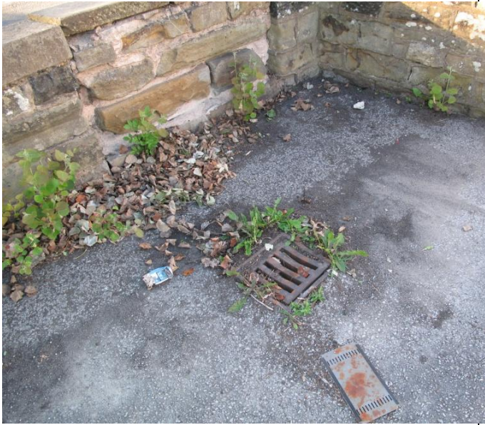
Gully in car park adjacent to boundary wall
