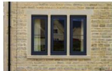
IMAGE 3 - INDICATIVE IMAGE OF RECONSTITUTED ART STONE WINDOW SURROUND. COLOUR TO BE SANDSTONE. WALLING NOT INDICATIVE OF RENDER FINISH.
