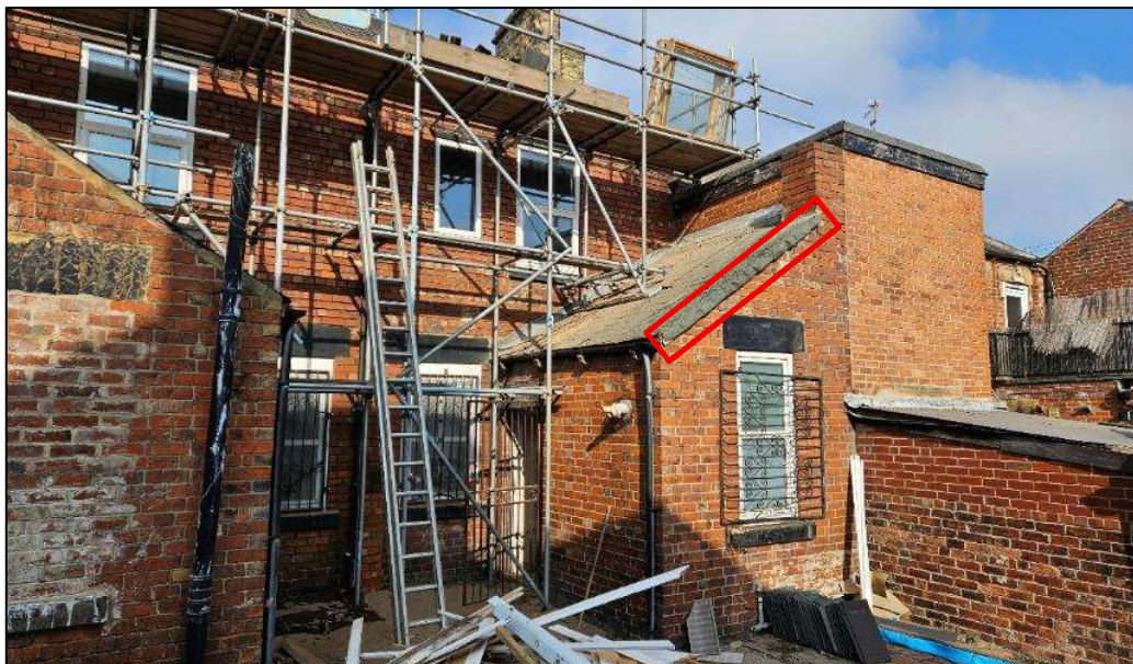
Plate 6. The roofing felt on the verge of the single storey section of the building which comprised the only potential roost feature present
