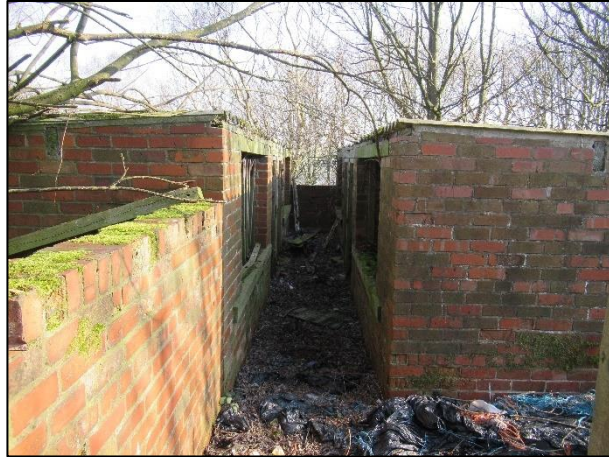
5.1.10.2. Photograph showing the open nature of the inside of the pig sties. These buildings are totally unsuitable for roosting bats.
