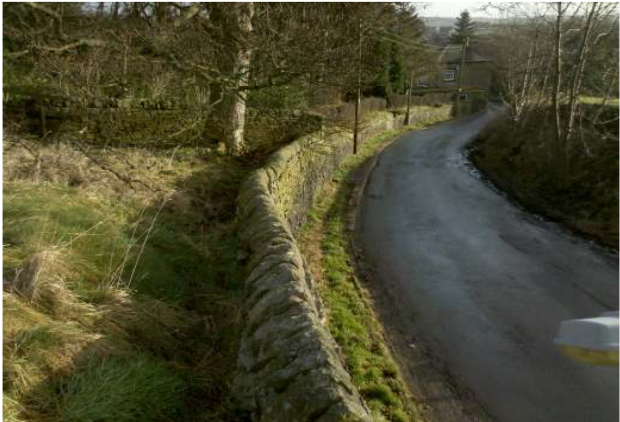
Photograph 11: View along Chapel Lane to east with stone retaining wall depicted on southern boundary
