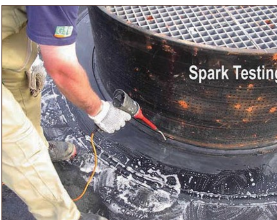
Figure A4.45 Spark testing (courtesy GSE Environmental)
