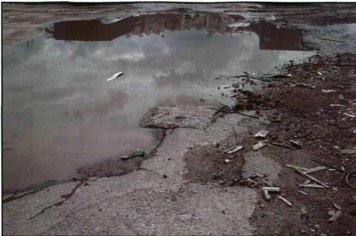
Photograph 7 Base of former obelisk and surface ponding.
