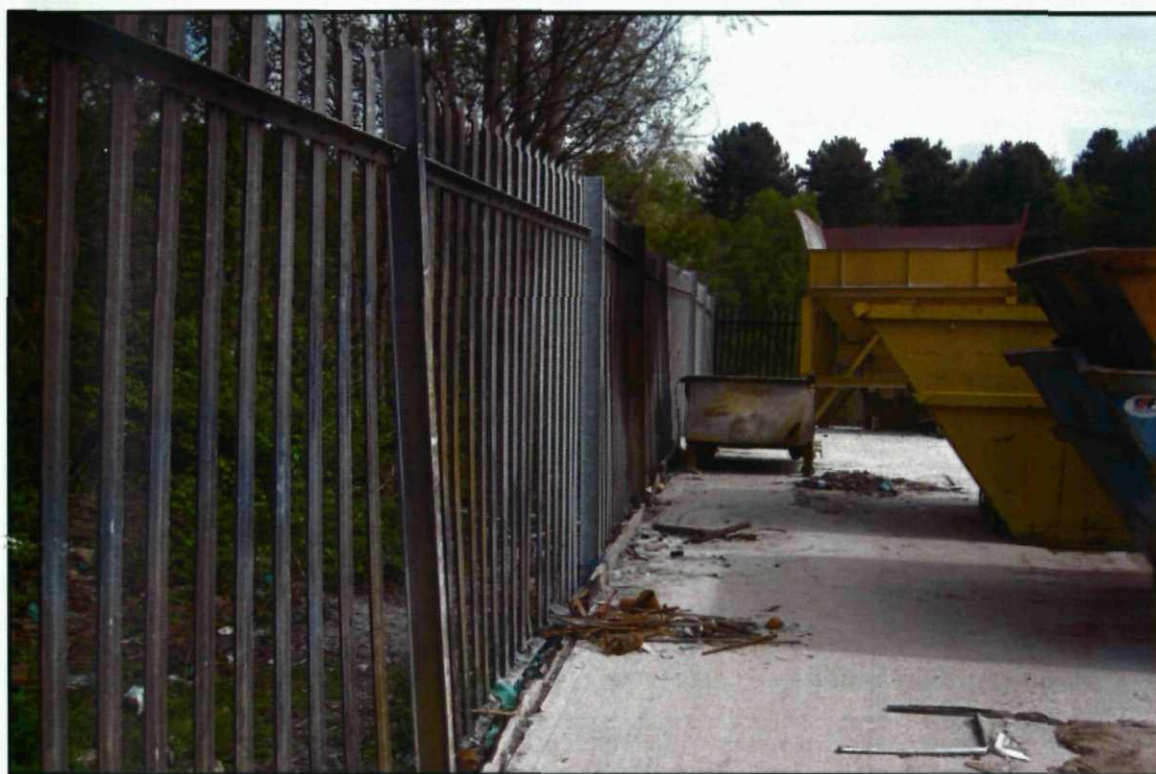
Photograph 12 Fire damage noted to security fencing.
