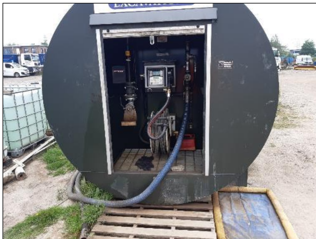
Figure 10: Red Diesel tank
