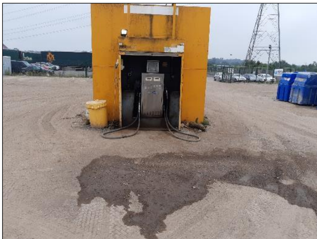
Figure 9: Road diesel tank with some stains
