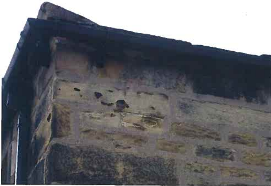
Current Plastic Guttering Supported on Crude Wooden Blocks
