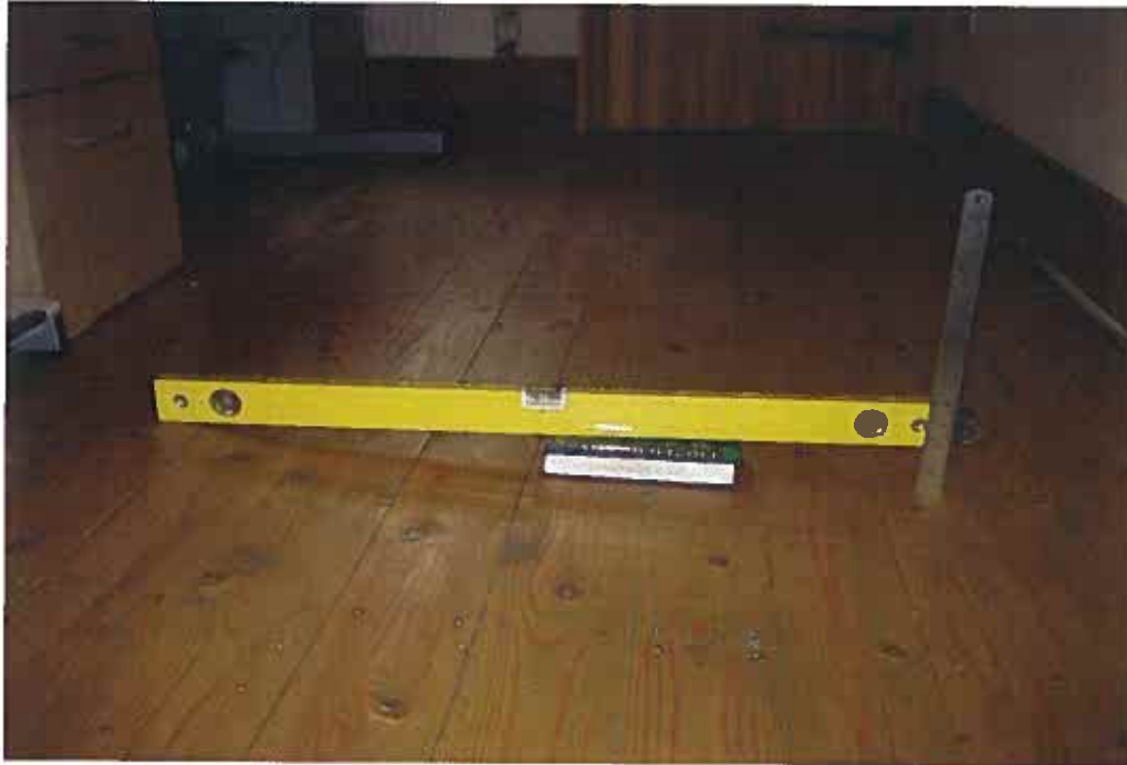
Current 3rd Bedroom Floor Illustrating Slope
