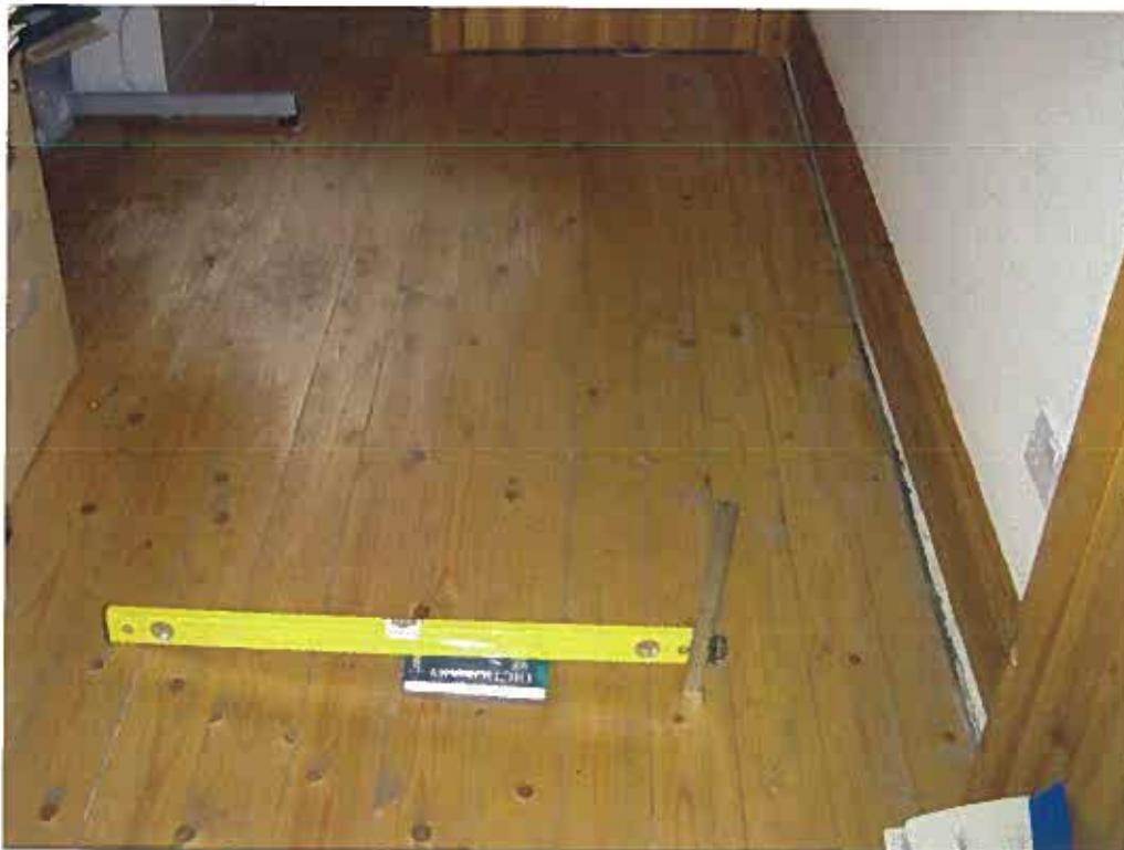
Current 4th Bedroom Floor Illustrating Slope and Modern Floor Boards
