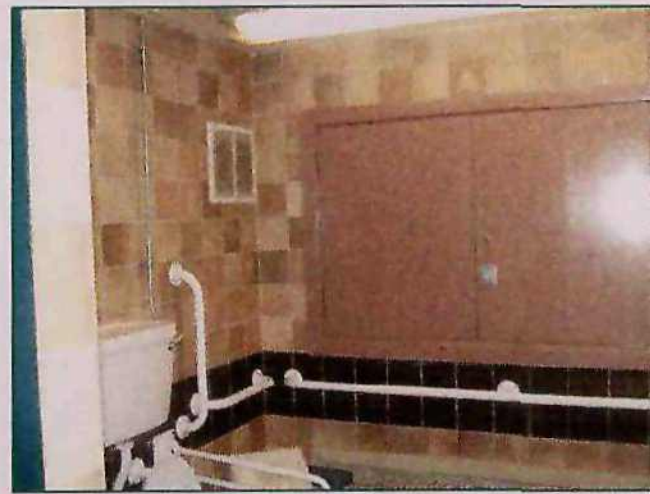
VIEW OF ELECTRICAL CUPBOARD IN DISABLED TOILET
