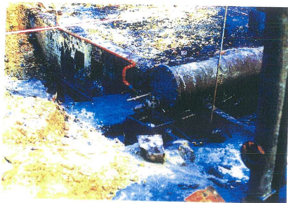
Figure 5.13 Contamination around the ram road sump.
