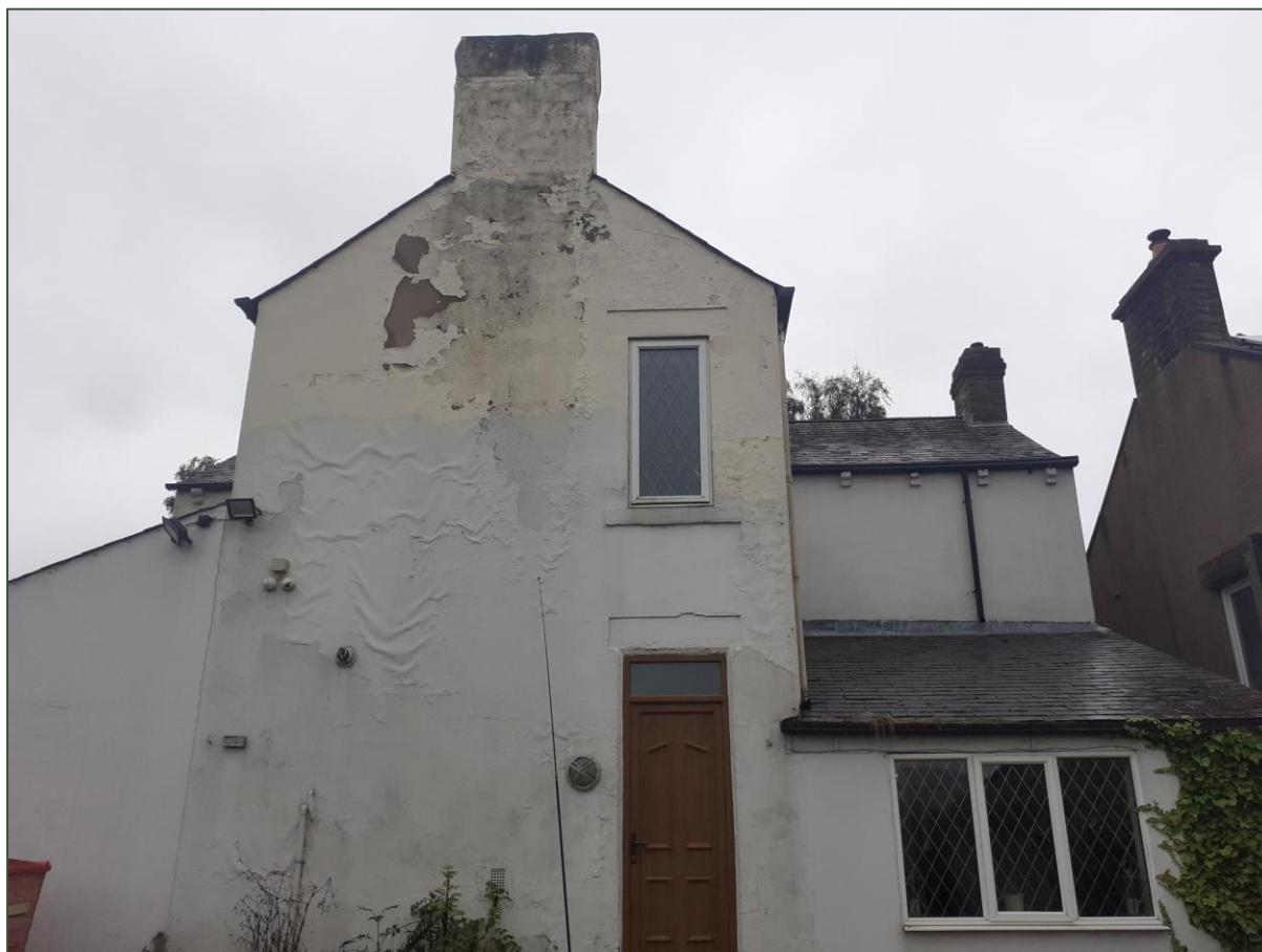
Plate 1: Rear (eastern aspect) of the property; proposals involve the replacement of the single storey extension to create a 'double gable', with a new extension in front (i.e. to the east).
