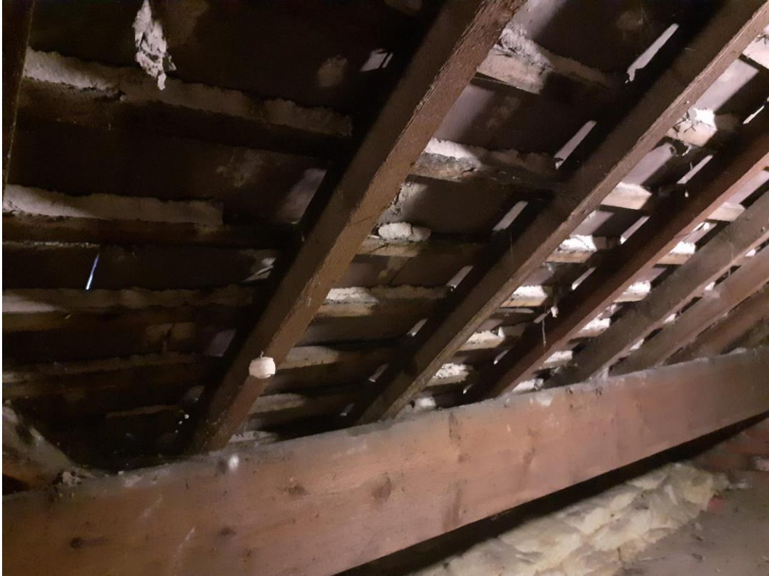
Plate 4: Underside of roof tiles (no membrane or sarking) above the single story extension pictured in Plate 3 (section with the chimney on right hand side of image).
