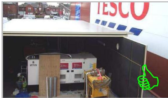
Generator within noise screen / enclosure
