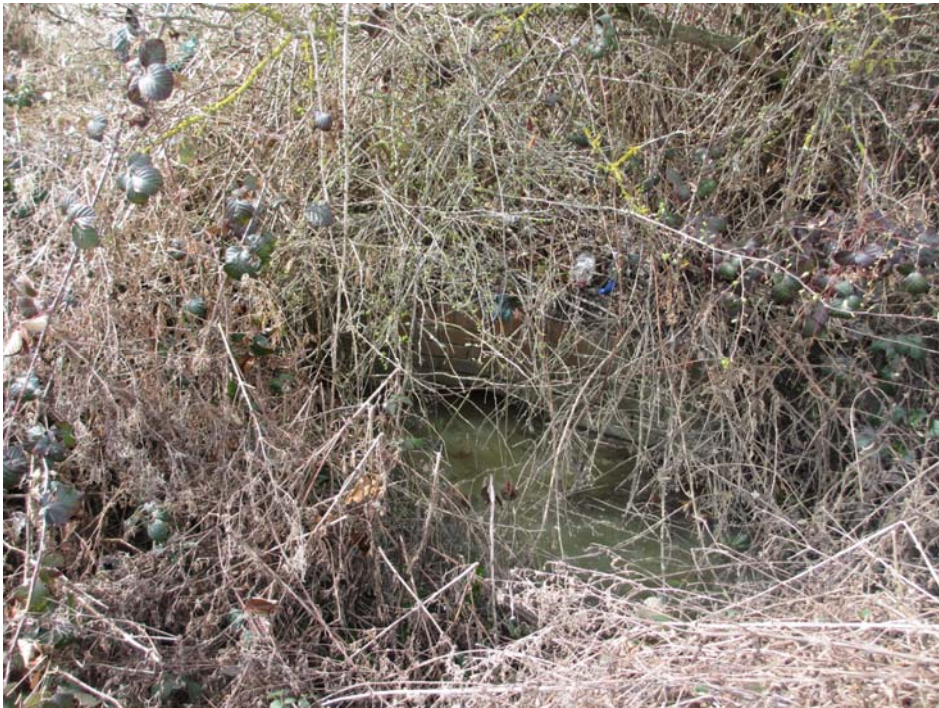
Northern Site – inlet headwall east of Woolley Colliery Road at field edge
