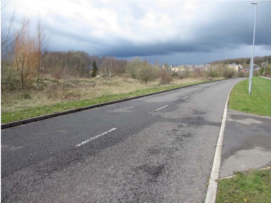
Northern Site – Low point in Woolley Colliery Road on overland flood route
