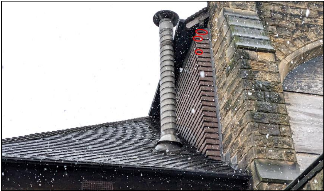
Plate 7. Crevices associated with hanging tiles on B2 (church hall)
