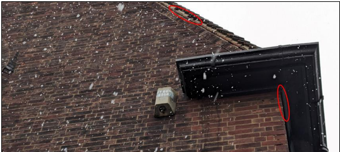
Plate 6. Gaps in verge mortar and between base of soffit and wall on B1 (church)
