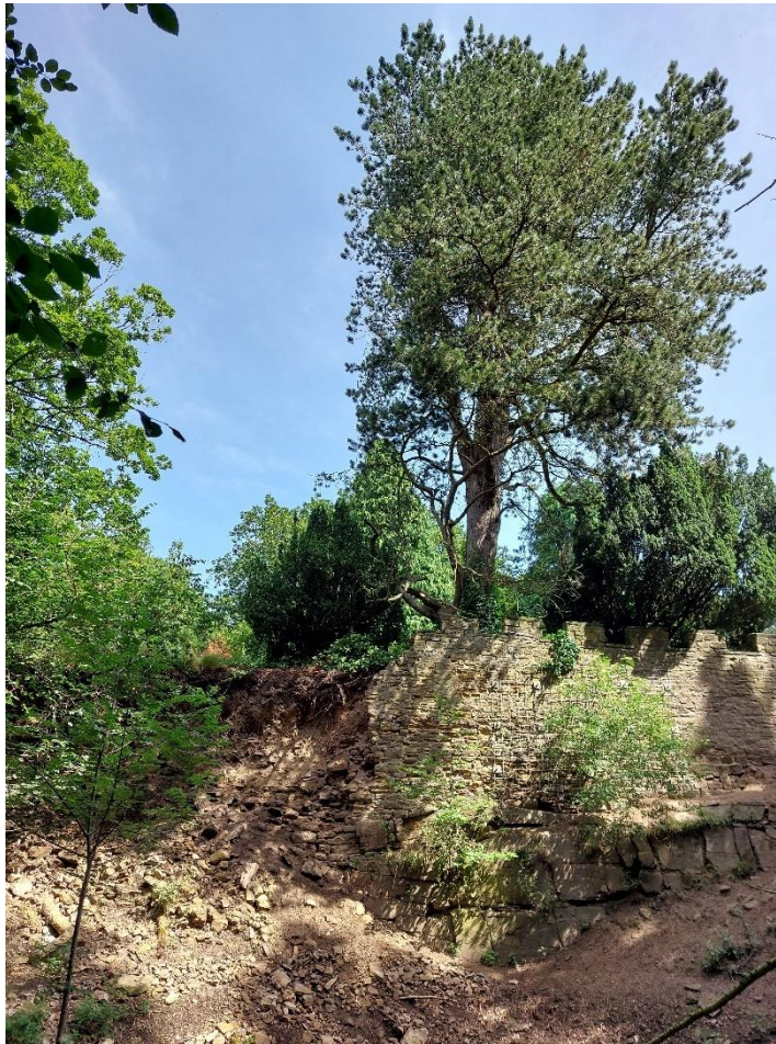
Plate 01: view of the collapsed and remaining sections of the Battlement wall, from the south. Trees 3873, 3947 and 3910 (left to right) are visible at the top of the wall. 15 July 2024.
