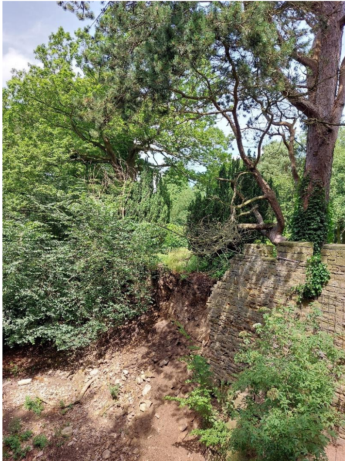
Plate 03: view of the collapsed and remaining sections of the Battlement wall, from wall-top level, from the southeast. Trees 3978, 3958, 3939, 3873 and 3947 (left to right) are visible. 15 July 2024.
