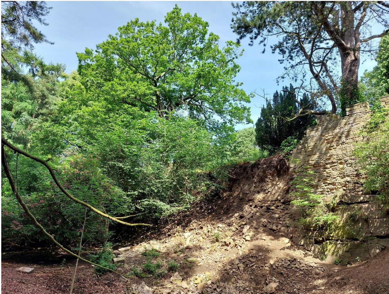
Plate 02: view of the collapsed and remaining sections of the Battlement wall, from the southeast. Trees 3978, 3958, 3875, 3873, 3947 and 3910 (left to right) are visible. 15 July 2024.
