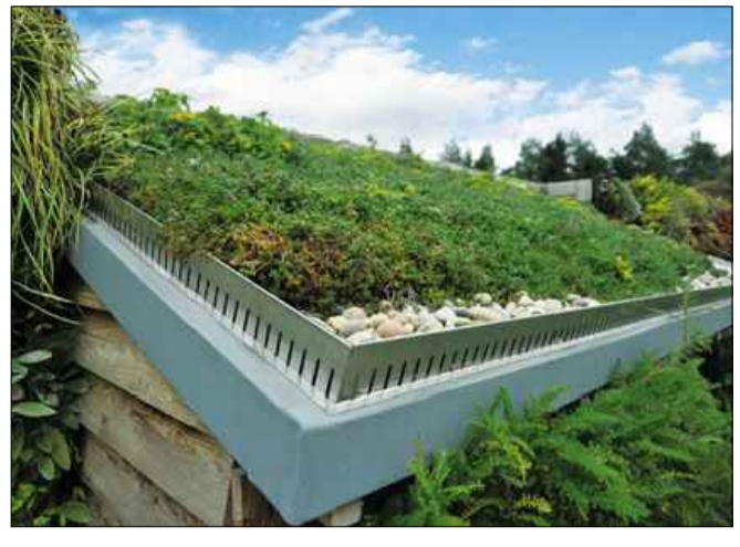
Example of ANS green roof when fully established
