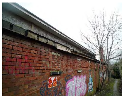
Figure 11. Eastern aspect of Building 4 with bricked up windows and broken guttering and fascia board.
