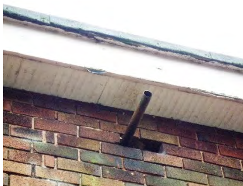
Figure 12. Northern aspect of Building 4 with gap in brick work providing PRF.
