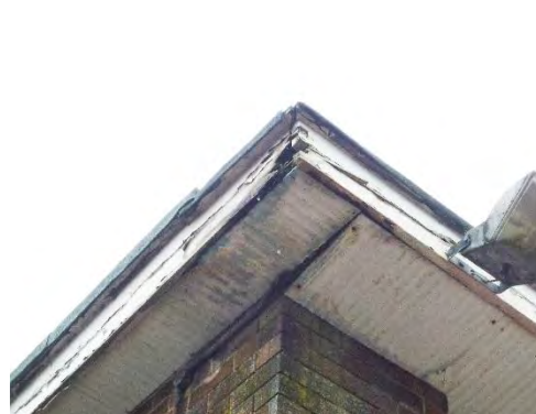
Figure 13. North-western corner of soffit box on Building 4 with gap in rotted fascia board and a dropped panel underneath the soffit box.
