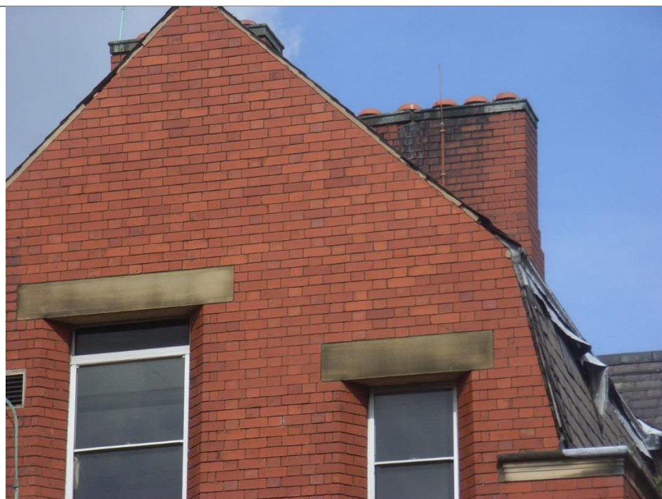
Plate 4: Building along eastern side of the site (TN4) viewed from west at roof level, showing lifted lead flashing and gaps between slates and brick wall, in which bats could roost.
