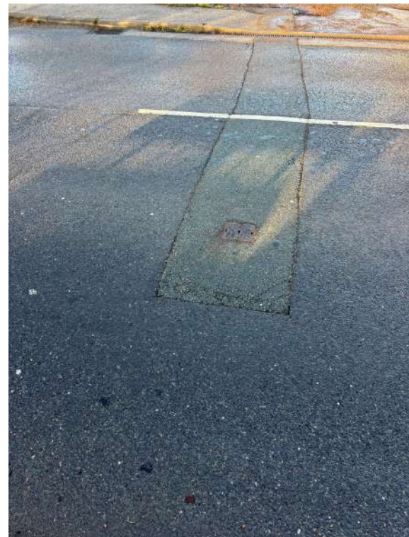
8 - Water meter lid & patch of tarmac to receive heavy traffic.
