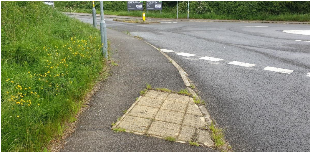
Figure 16 - Tactile paving on southern footway on east leg of mini roundabout.
