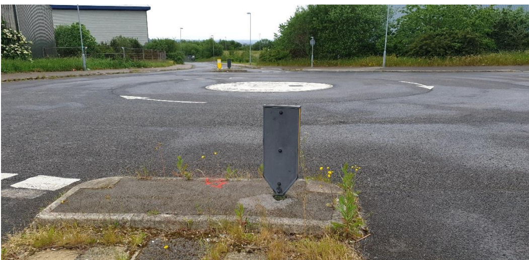
Figure 24 - View from pedestrian island on southern leg. Heavy vegetation in kerb lines/tactile paving.
