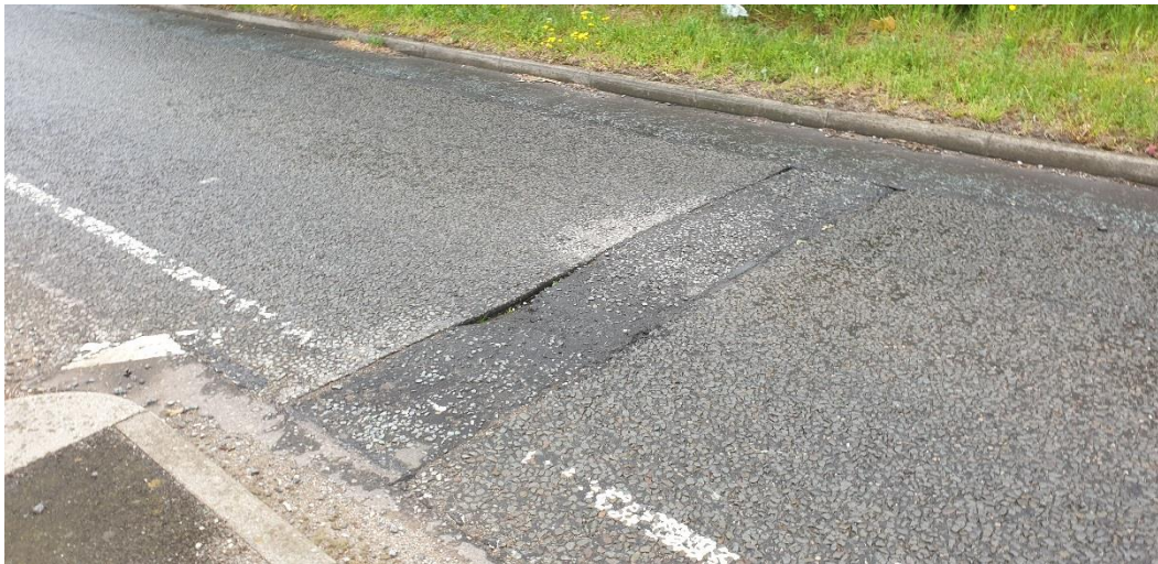
Figure 2 - Failed reinstatement on Ryecroft Bank to the north of junction with Ashroyds Way.
