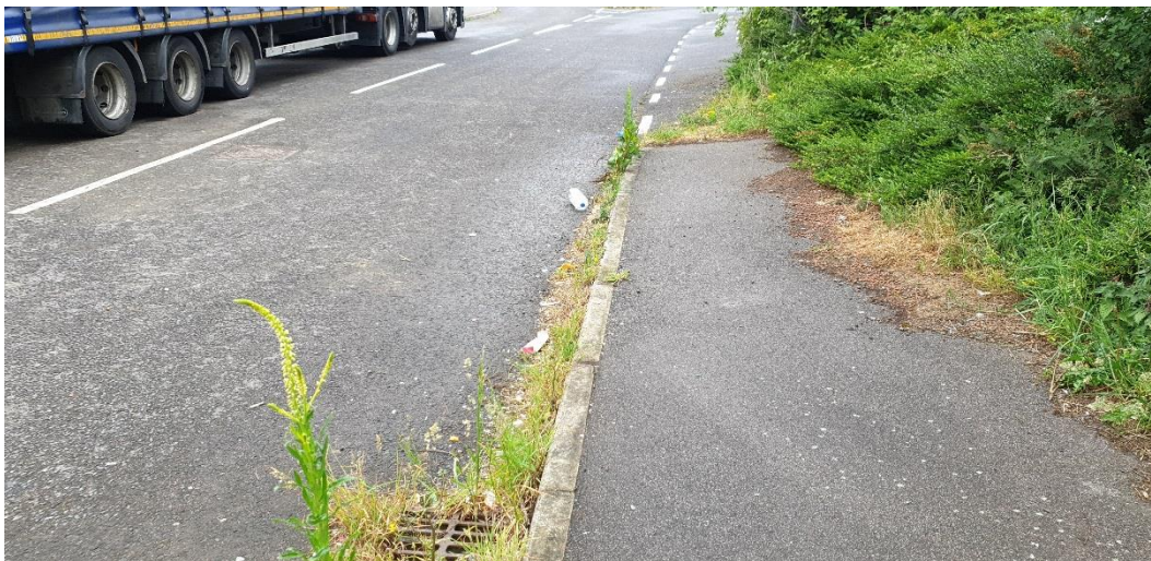
Figure 41 - Growth in channel linem encroaching back of footway and over tactiles.
