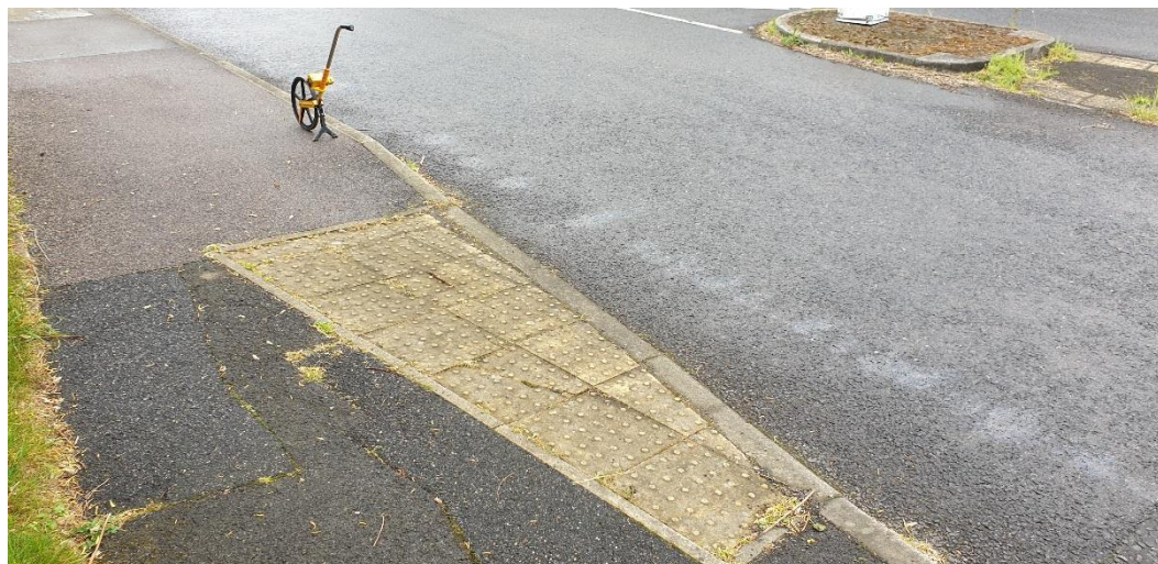
Figure 6 - Tactile crossing at entrance to site. Pavers cracked but not rocking.
