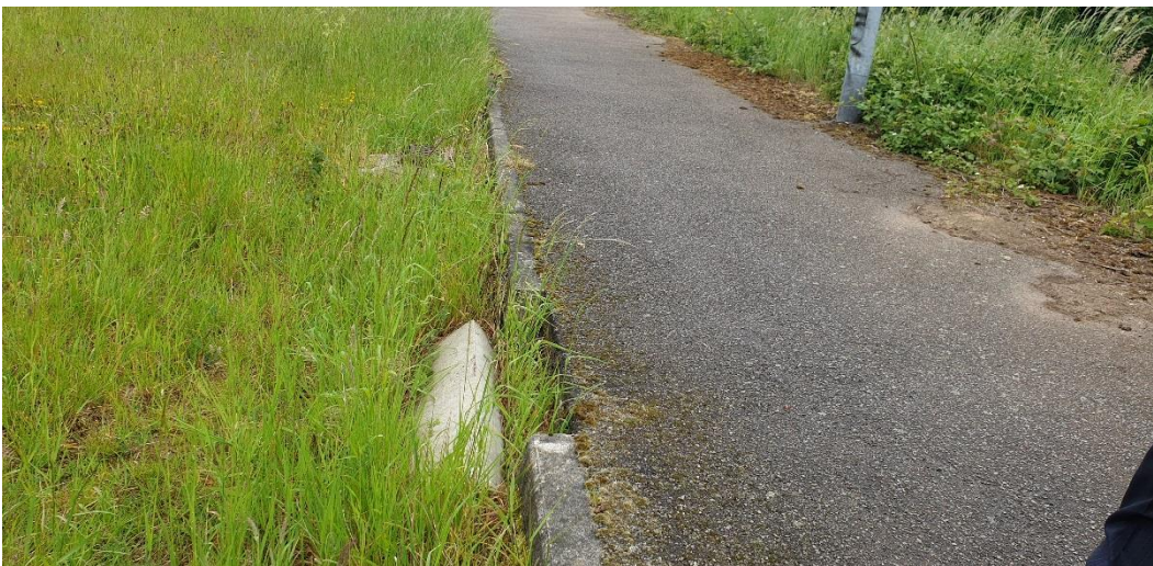
Figure 51 - One kerb has dislodged. To be replaced in S38 works.
