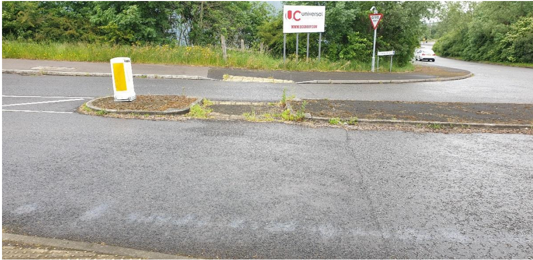
Figure 7 - View across pedestrian crossing. Heavy vegetation in channels and against kerbs.
