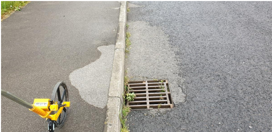
Figure 13 - Some minor cracking in surface course around gully.
