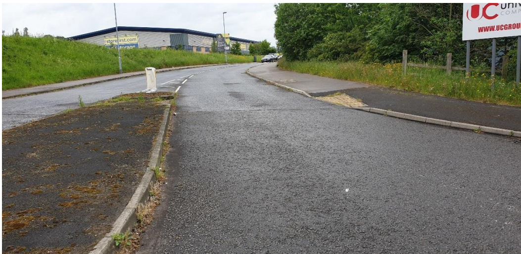
Figure 5 - View west of outbound lane. Some minor chipping loss in surface course.
