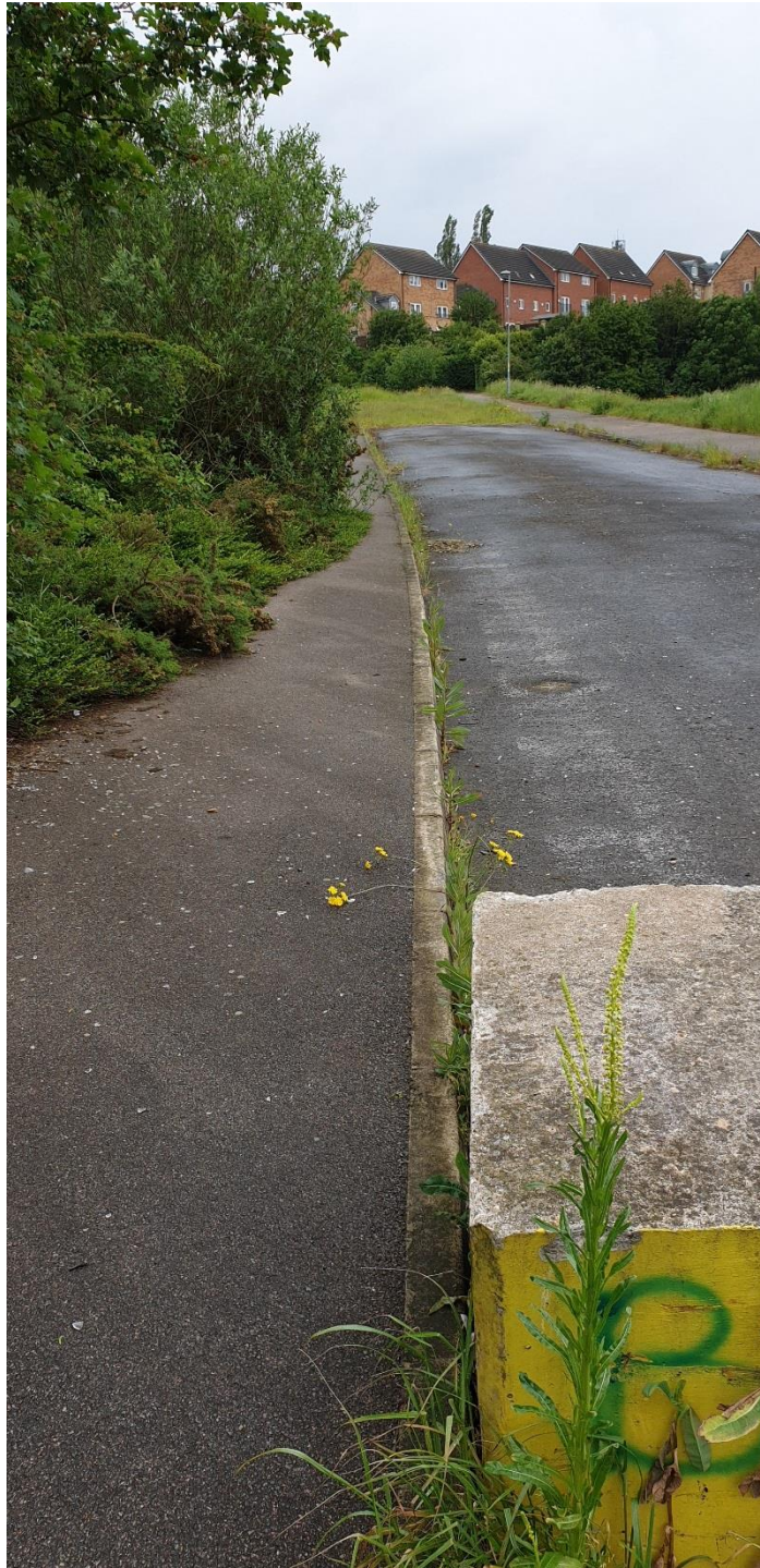
Figure 44 - Eastern channel looking south from concrete blocks. Vegetation encroaching over footway.
