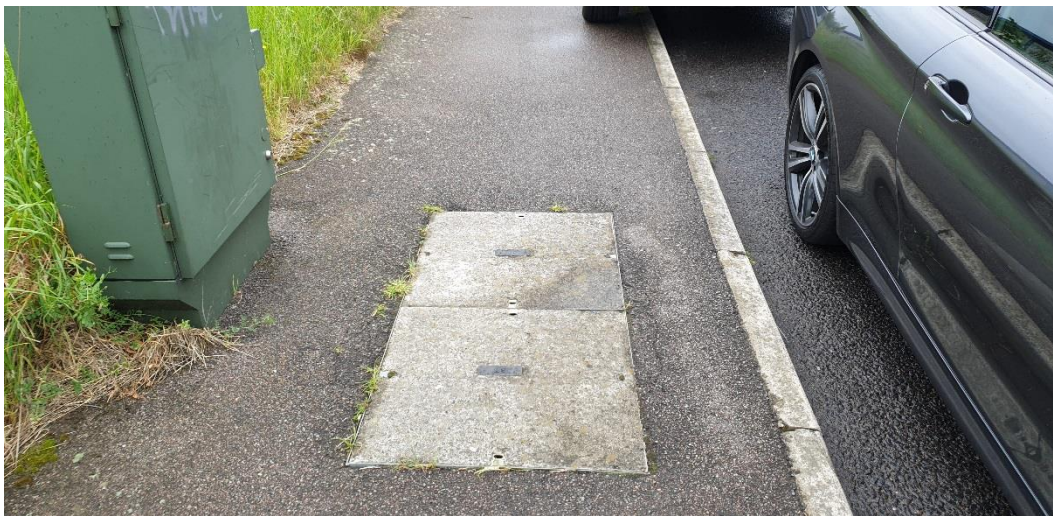
Figure 9 - BT chamber in southern footway.
