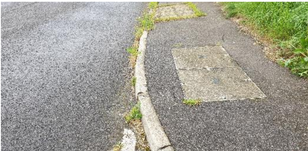
Figure 27 - Chipped kerbs on western side of southern leg off mini roundabout adjacent BT box.
