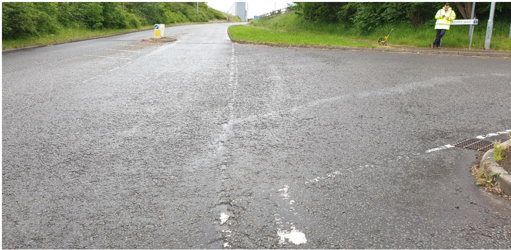
Figure 4 - View north of westbound lane into Ashroyds Way. Some minor chipping loss in the surface course. All junction lining is worn out.
