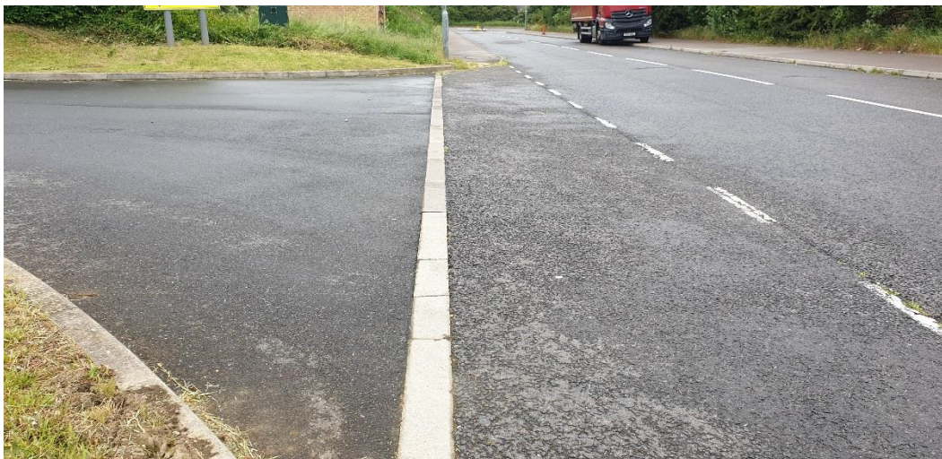
Figure 11 - Existing demarcation channels at rear of Highway boundary. Some channel blocks are loose and rocking.
