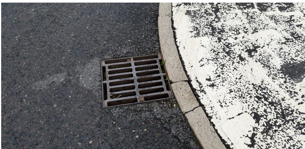
Figure 21 - Loose kerbing adjacent gully on island.
