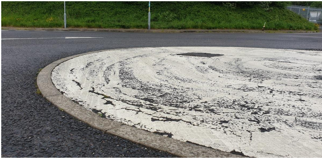
Figure 33 - Depression in mini-roundabout surfacing.
