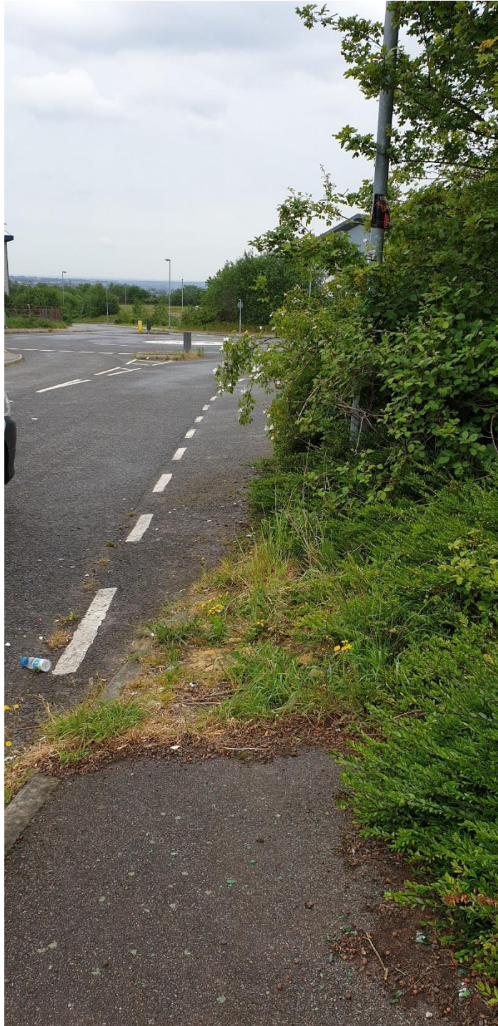
Figure 45 - Tactile crossing across access. Vegetation encroaching.
