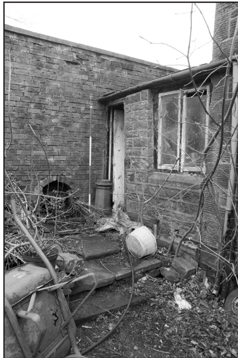
Photograph Number: 2 Reference: RLHS_002 Description: Boiler house to the south side of the Lodge Direction: NW
