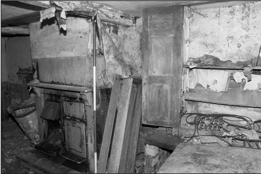
Photograph Number: 35 Reference: RLHS_035 Description: Range and cupboards in Cottage 7 Direction: S
