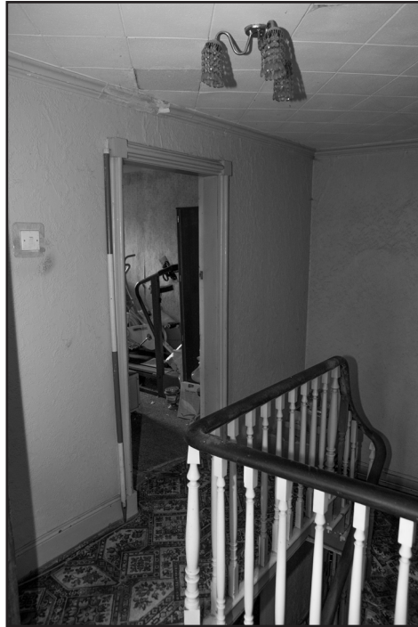
Photograph Number: 9 Reference: RLHS_009 Description: First-floor landing in the Lodge Direction: NW
