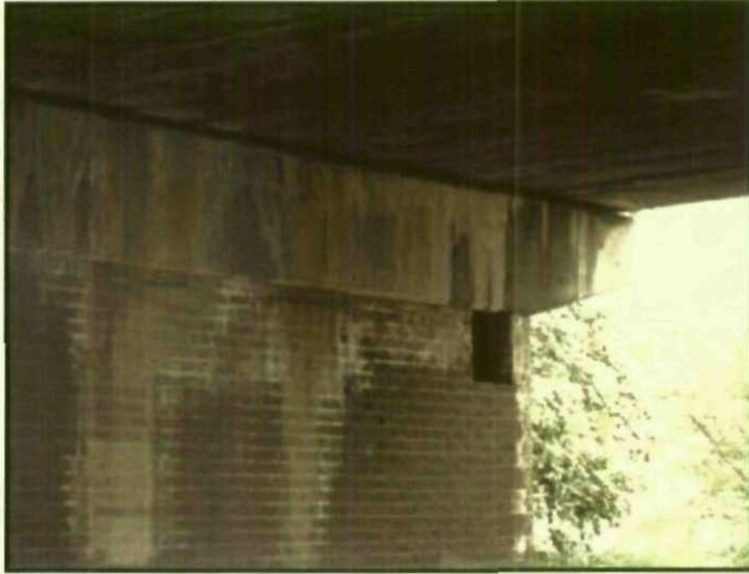
Photograph 1. Gaps within the bridge that may be suitable for roosting bats.
