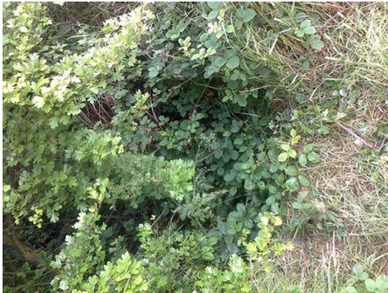
Photo 8. Vegetation filled drain north of TN1
