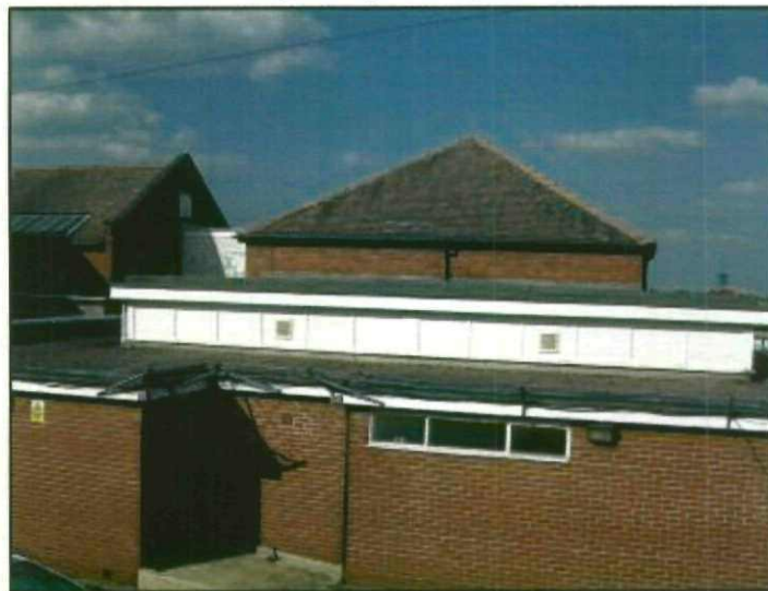
Plate 5 Barnsley College Honeywell –flat roof sections to north western corner of building
