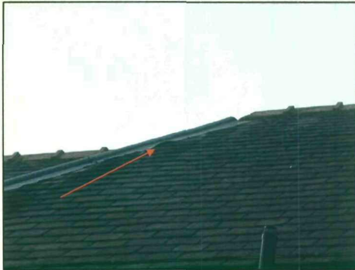
Plate 16 Gaps beneath lead flashing on main Barnsley College Honeywell Building
