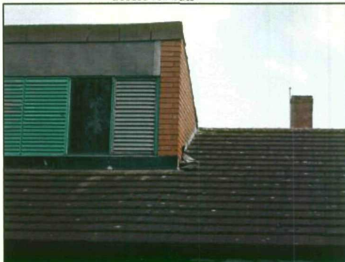
Plate 18 Potential bat access points beneath lead flashing and air vents in substation building
