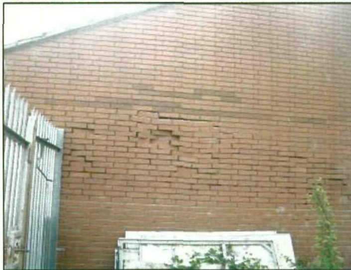
Plate 17 Gaps within the brickwork of the substation wall, which may provide potential access for bats
