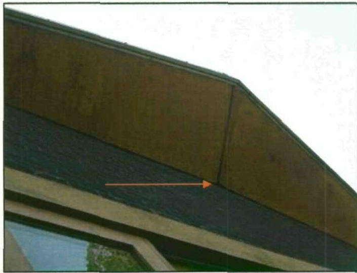
Plate 15 Apparent gaps (thumb width) into wooden soffit potentially suitable for bats
