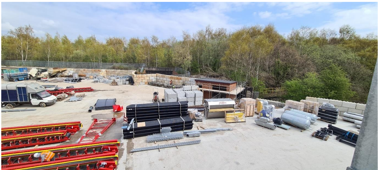
Figure 3. Photograph of the site's yard area (looking east) from the filter press element of the aggregate washing plant
