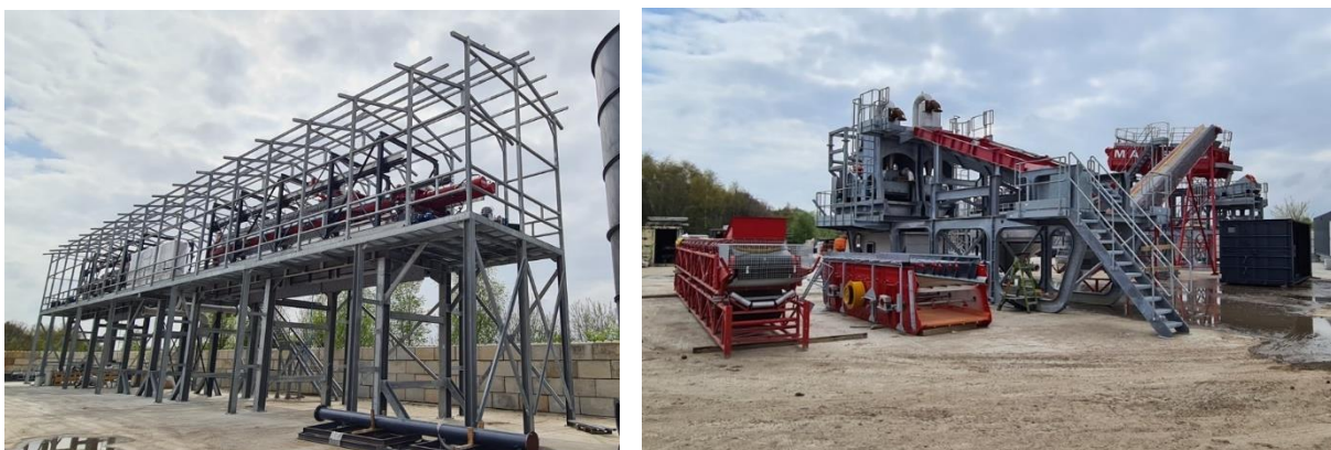
Figure 4. Photographs of the filter presses' supporting structure (left hand side) and washing system (right hand side)
