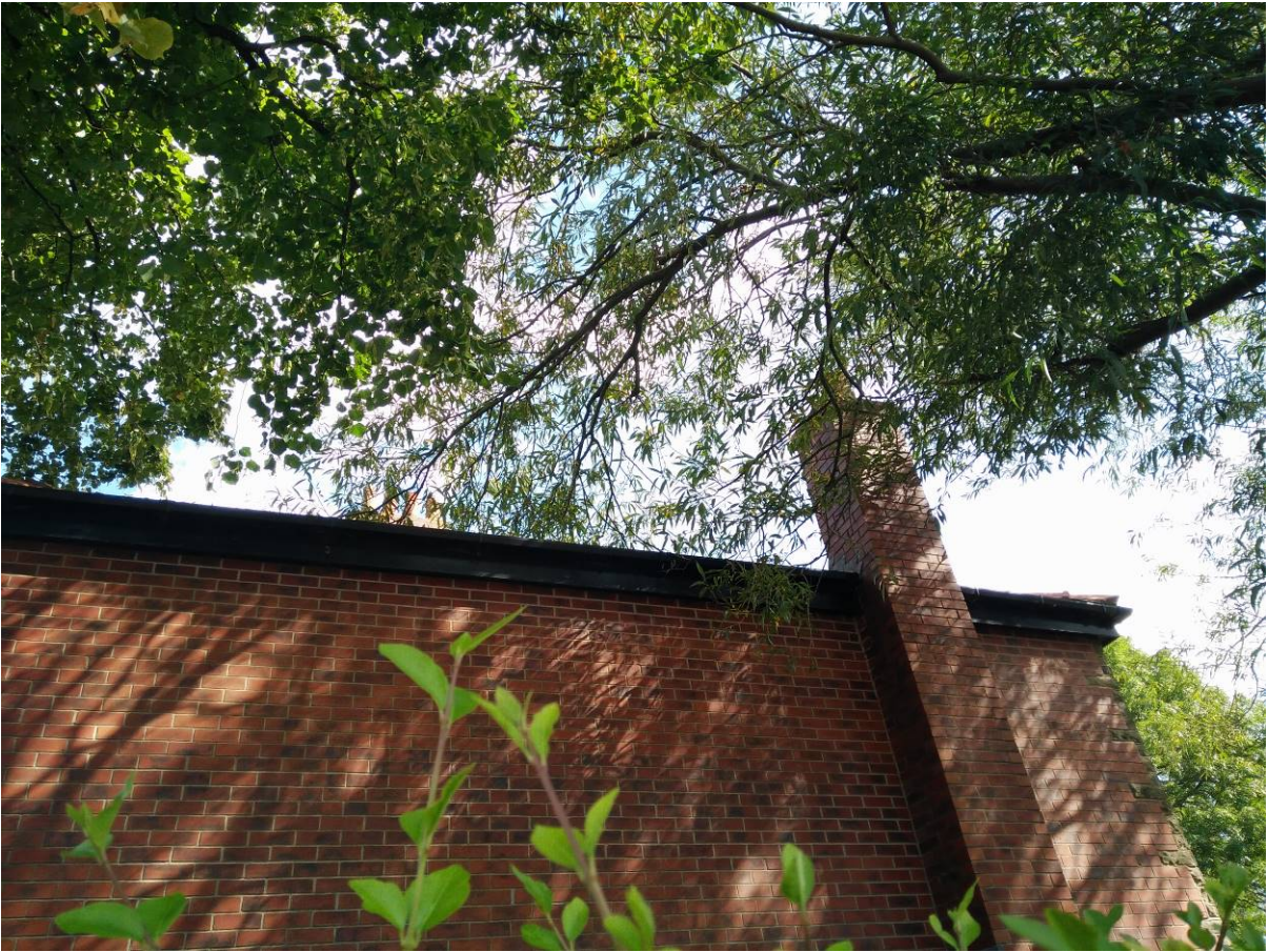
Canopies of Tree No's 6 and 7 Touching the Roof/Chimney of the Property
