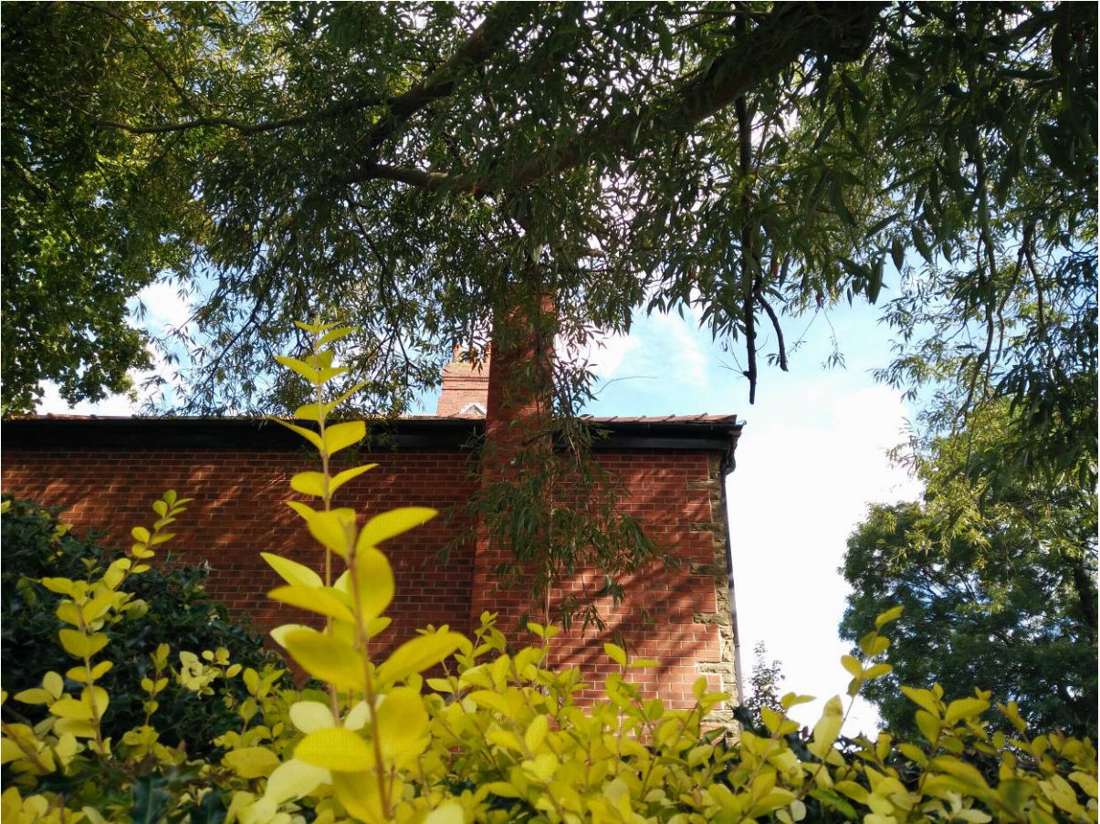
General View of the Canopy of Tree No 6 Touching the Roof/Chimney of the Property
