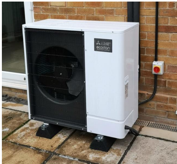
Air source heat pump condenser
