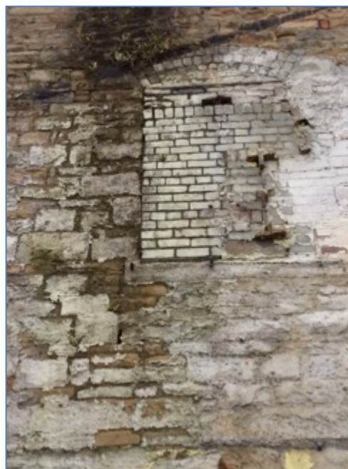
Photograph 35. External view of some of the cavities and gaps in mortar of B10 (TN11)
