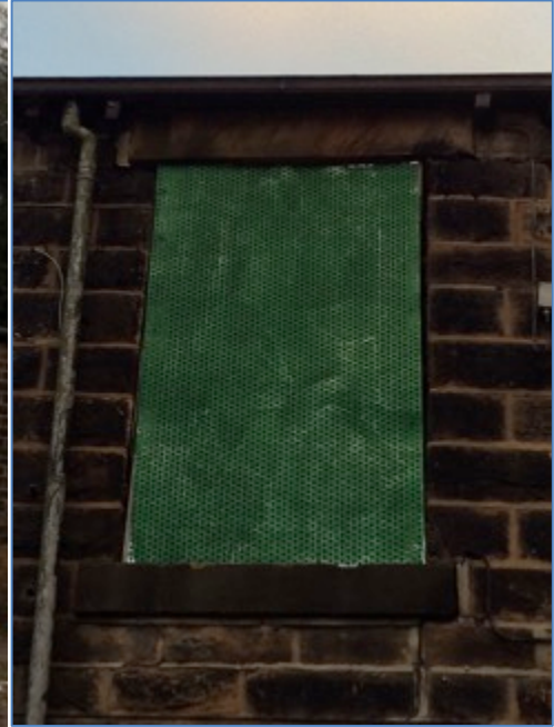
Photograph 39. Crevices between stonework and under lintels, B18 (TN10)
