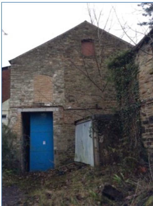
Photograph 32. Northwest gable of B10 (TN11), showing lintel (4 sections deep) above the blue door; location of live bats
