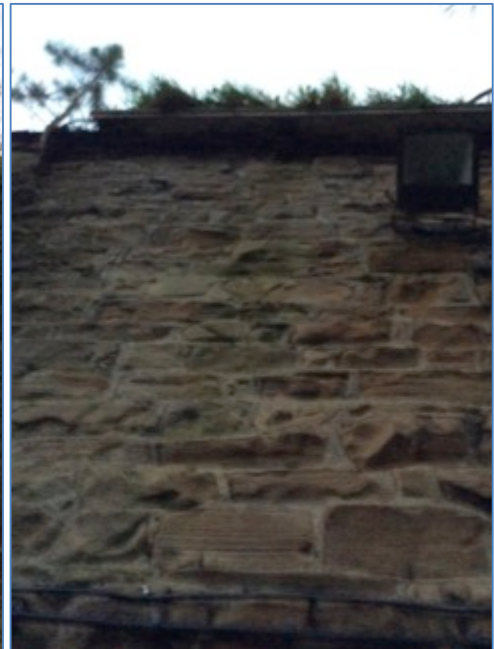
Photograph 37. Gaps under guttering at B9 (TN13), rear side.
