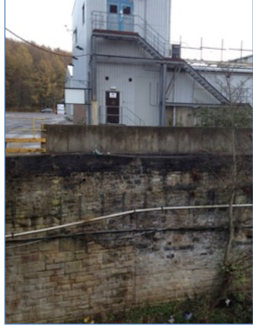
Photograph 16. River Don wall (TNI) as viewed from the south side of the bridge, facing north. B19 in the background.
