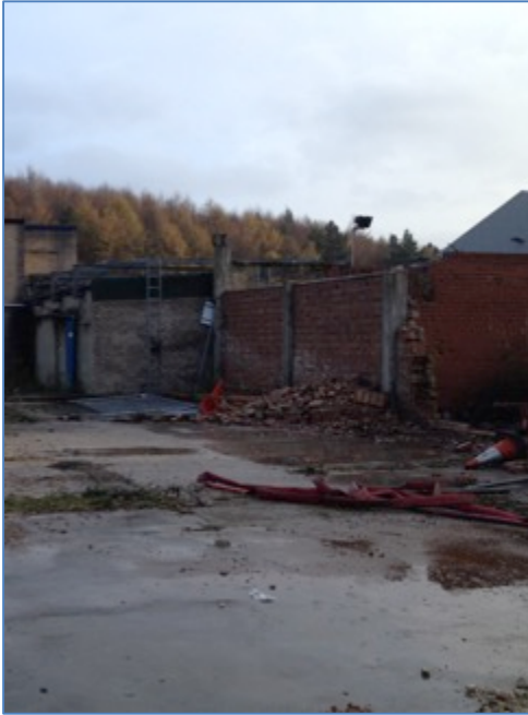
Photograph 3. Brick rubble pile next to derelict brick structure B4, at TN4
