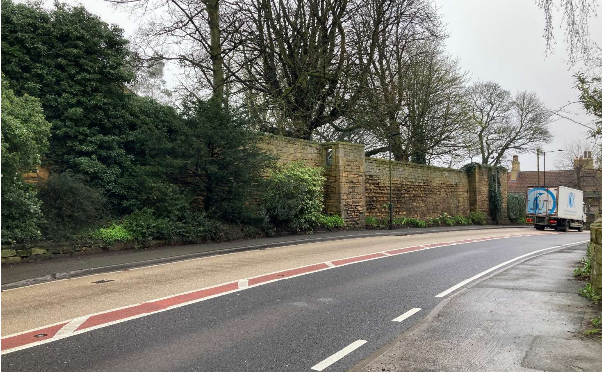
Plate 7 - Listed Wall from the north-east, road condition visible
