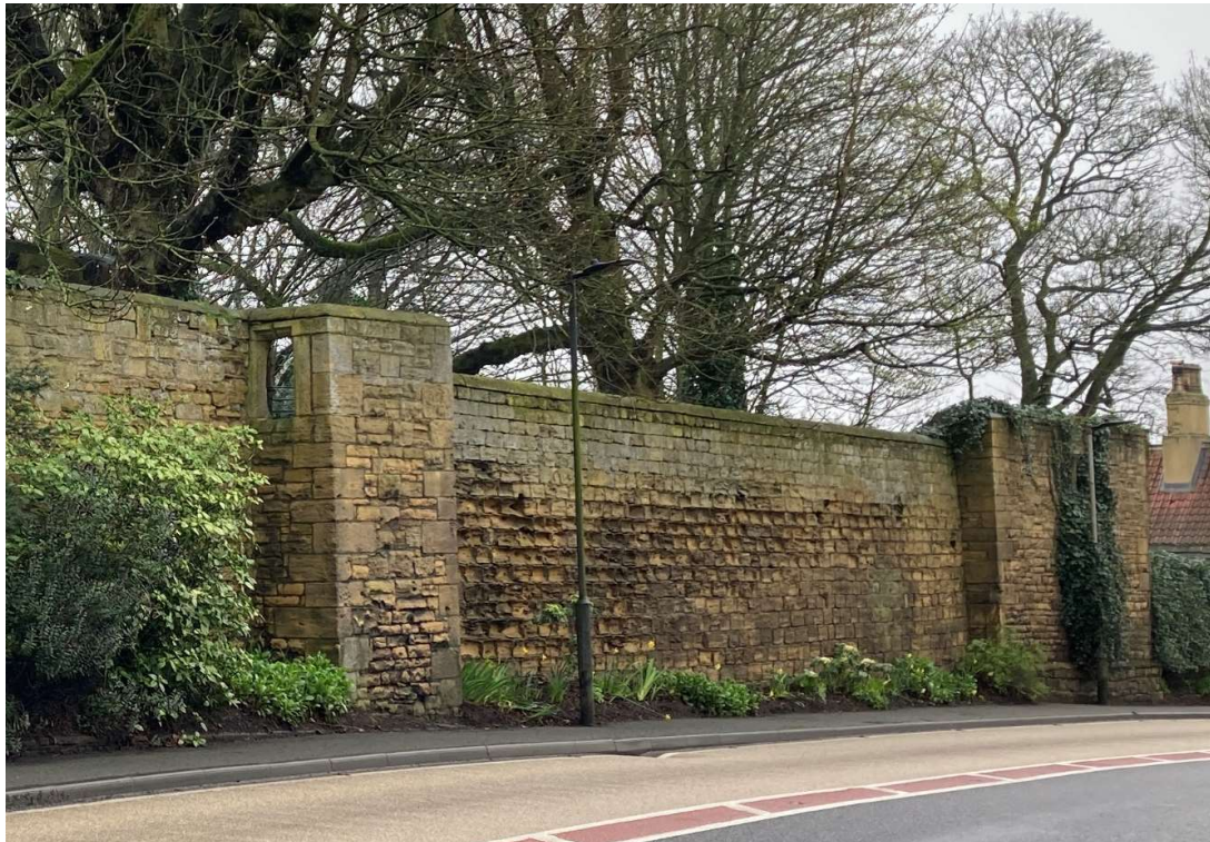
Plate 3 - Large area of weathered stone.
