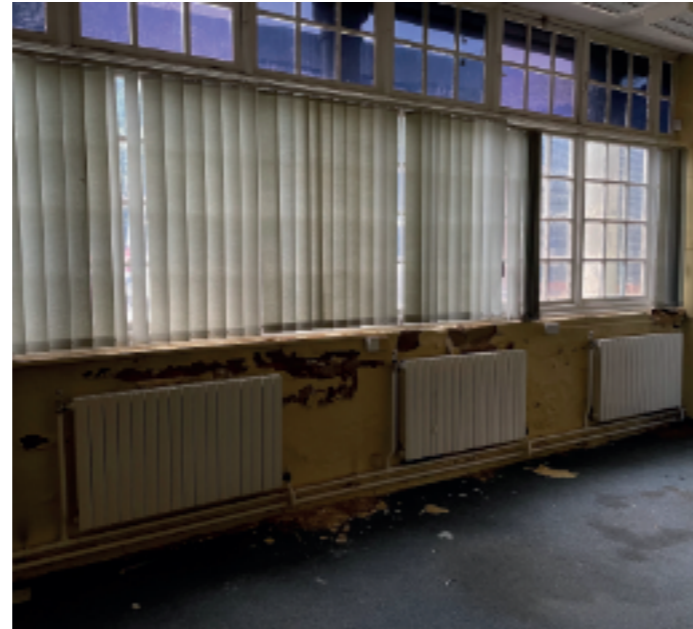
Western façade; severe water damage
