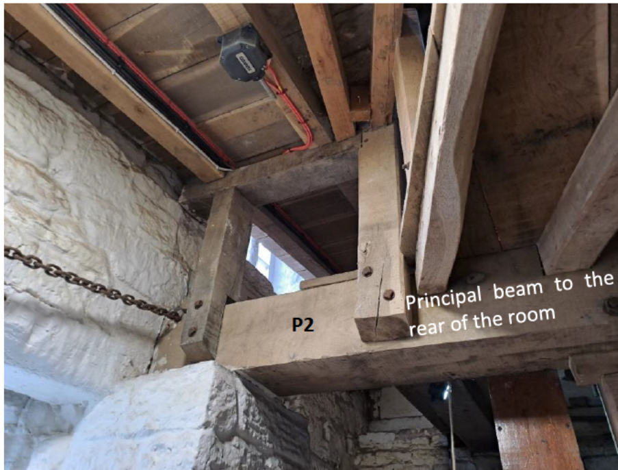
5 Ground-floor level - Milling Room 3. Timber posts supporting the ramp and connected to principal beam at the rear. Timbers generally in good condition. Minor corrosion to fixings. In average 17% relative humidity.
