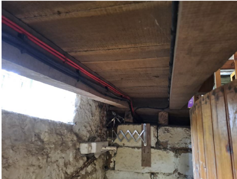
3 First-floor level - Milling Room 2. Underside of existing ramp. Timbers generally in good condition.
