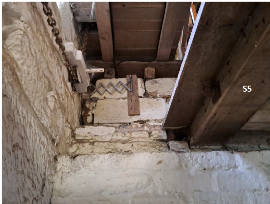
6 Ground-floor level - Milling Room 3. View of upper floor timber support beam S5.
