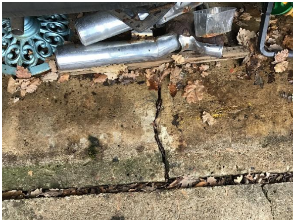
Historic cracking to garage floor slab
