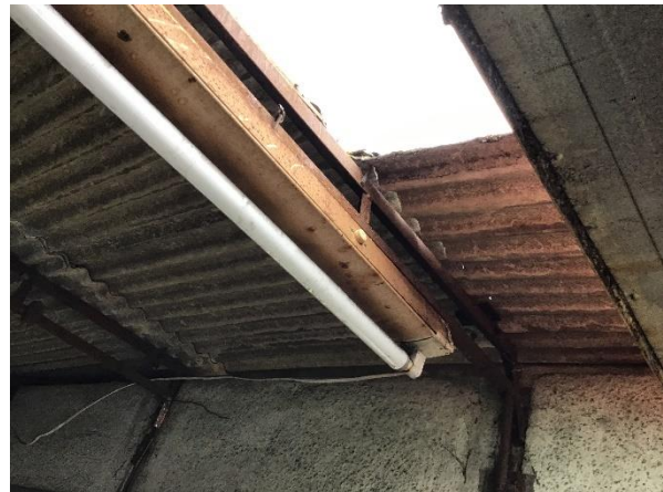
Missing asbestos roof sheet to middle of the garage
