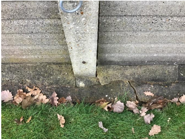
Cracking at the right-hand junction of the rear extension
