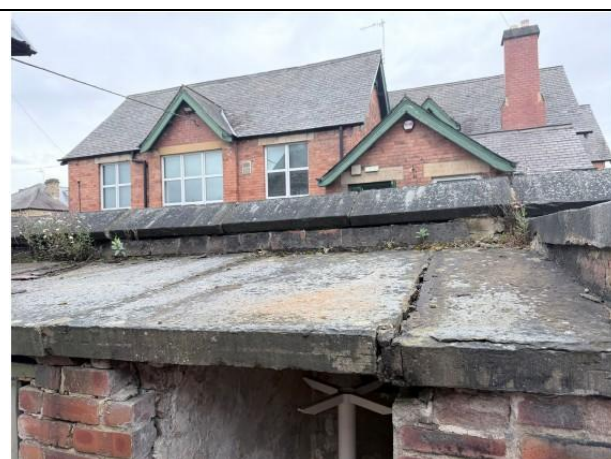
Photo 5 – Condition of stone slab roof and lack of support
