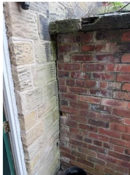
Photo 3 – Movement and separation between outbuilding and main structure
