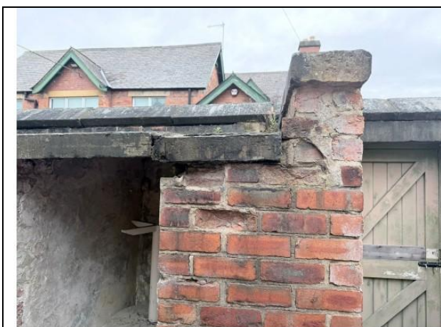
Photo 4 – Displacement and rotation of brickwork wall
