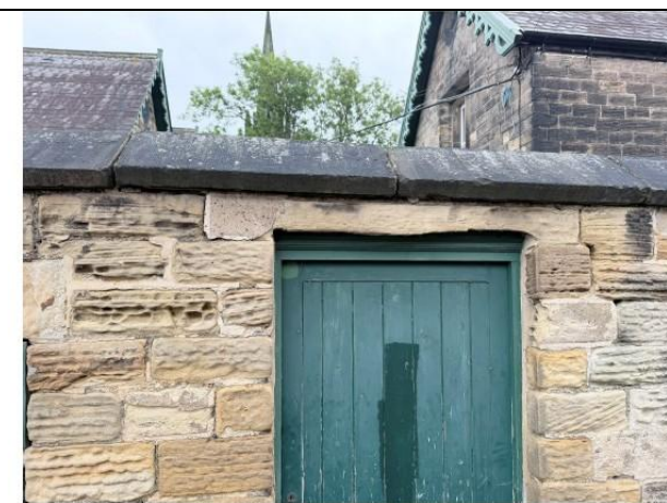
Photo 7 – Weathered stone lintel to access opening
