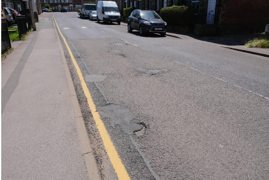
Photograph 14: Existing road surface on Hoyle Mill Road just south of junction with Foster Street.
