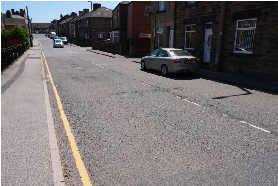
Photograph 13: Existing road surface on Hoyle Mill Road just south of junction with Victoria Street.
