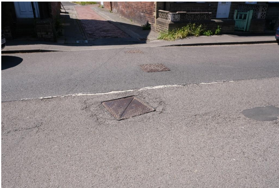
Photograph 15: Existing road surface on Hoyle Mill Road just south of junction with Foster Street.
