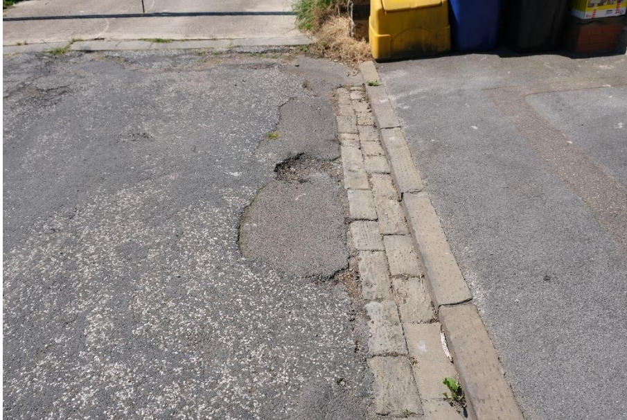
Photograph 2: Potholes adjacent to footway on the north flank of Hopewell Street.
