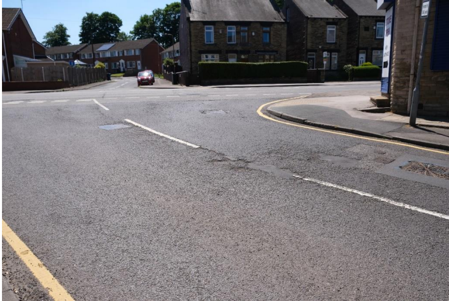
Photograph 16: Existing road surface on Hoyle Mill Road just north of junction with A635 Doncaster Road.
