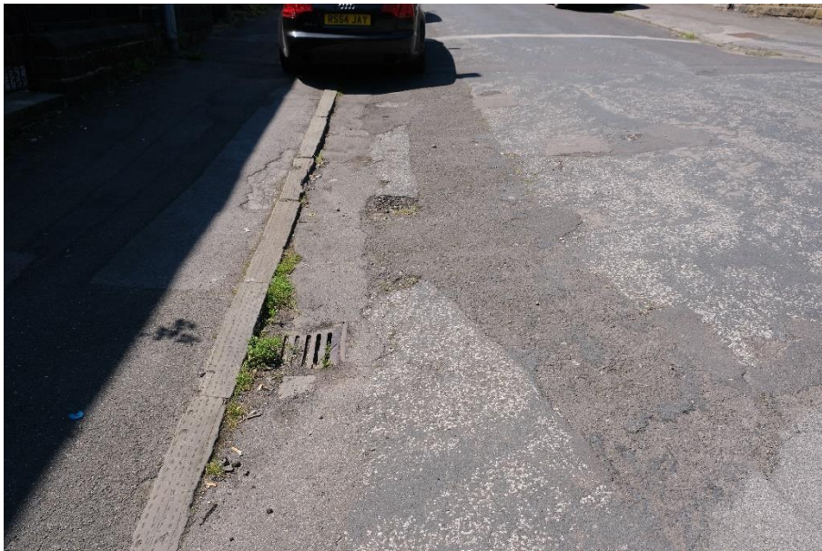
Photograph 7: Existing road surface and gulley on southern flank of Hopewell Street.
