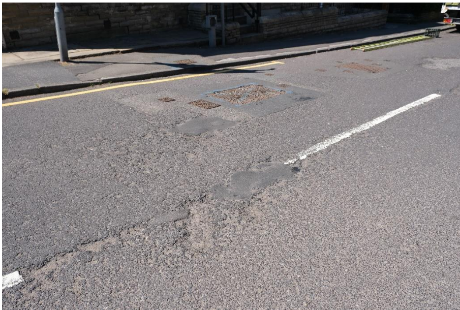
Photograph 17: Existing road surface on Hoyle Mill Road just north of junction with A635 Doncaster Road.
