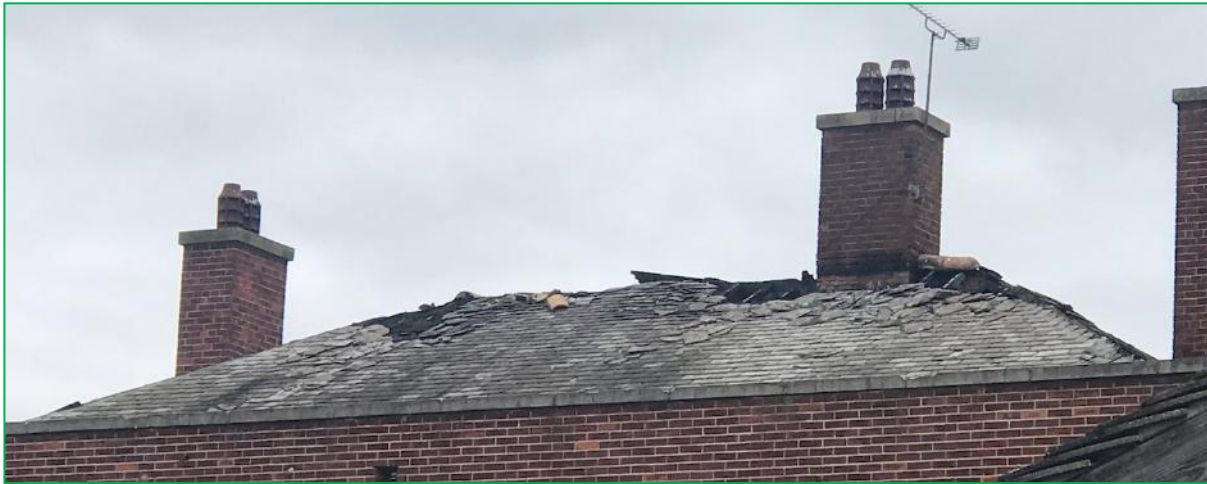
Showing lifted and missing slates on the west elevation of the building
