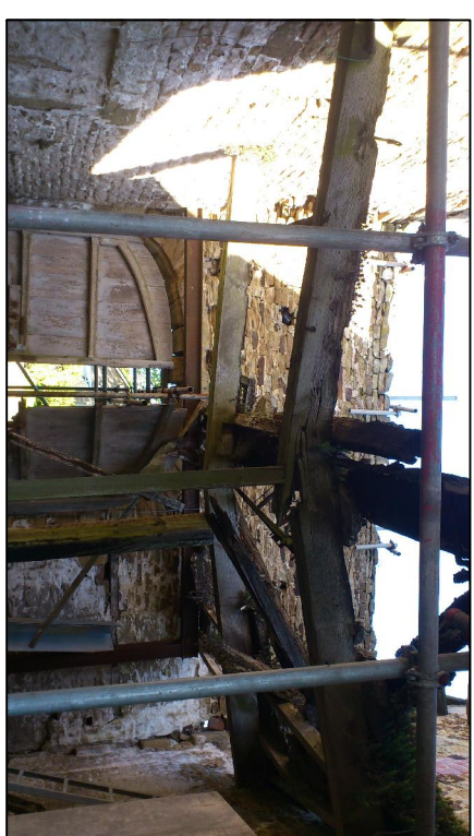
PICTURE B ENTRANCE AREA AND REMAINS OF STRUCTURAL MASONRY AND TIMBER FRAME PROPPING
