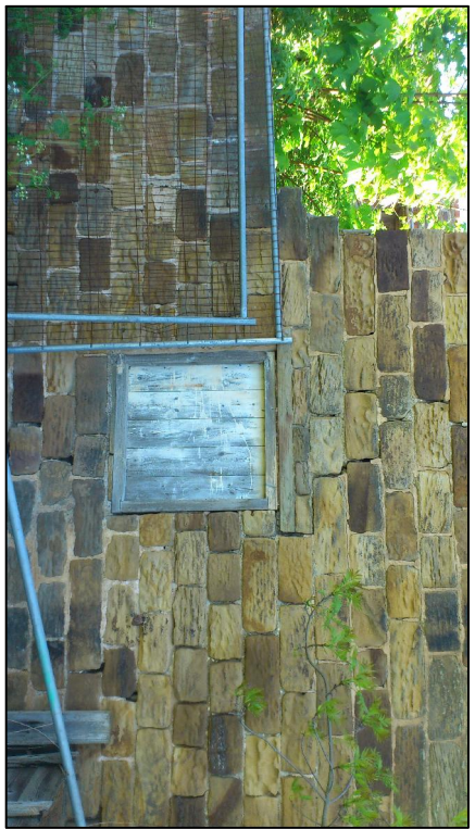
PICTURE U SHOWING MISSING SECTION OF EXTERNAL WALL
