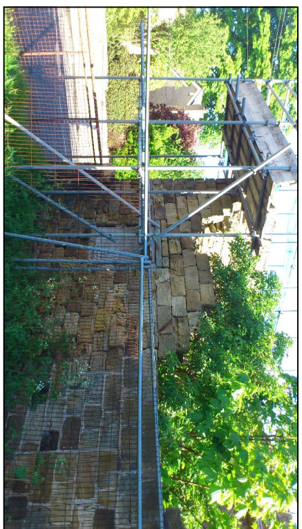
PICTURE V SHOWING MISSING SECTION OF EXTERNAL WALL
