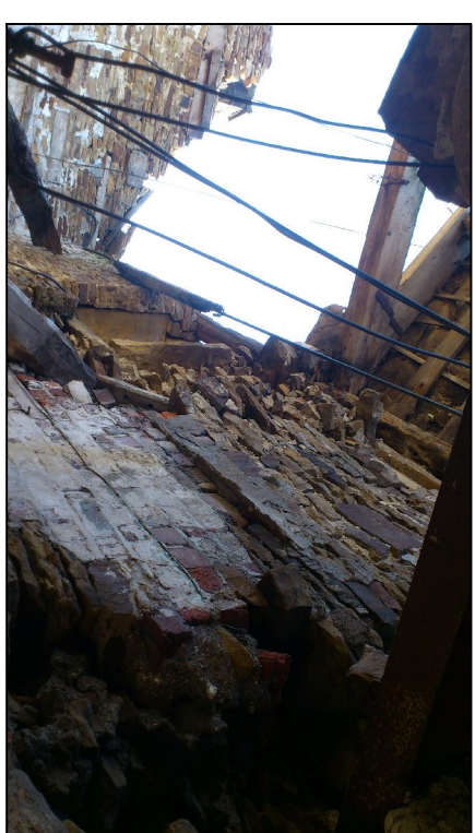
PICTURE G SHOWING DETEIORATION OF SUPPORTING MASONRY TO ROOF TRUSS
