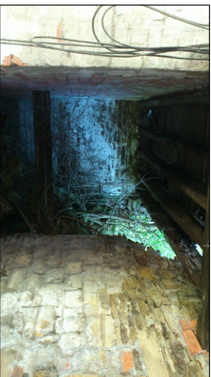
PICTURE U SHOWING MISSING SECTION OF EXTERNAL WALL
