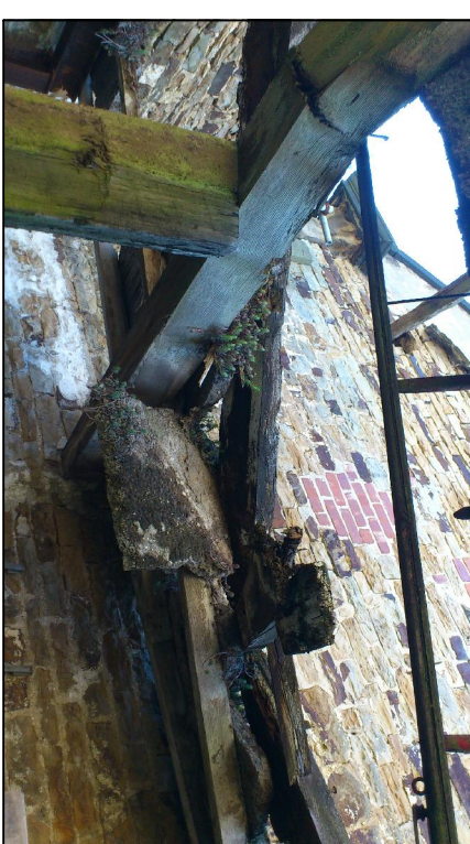
PICTURE A SHOWING FRACTURED TIMBER FLOOR BEAM AND STRUCTURAL FLOOR COLLAPSED INTO BUILDING
