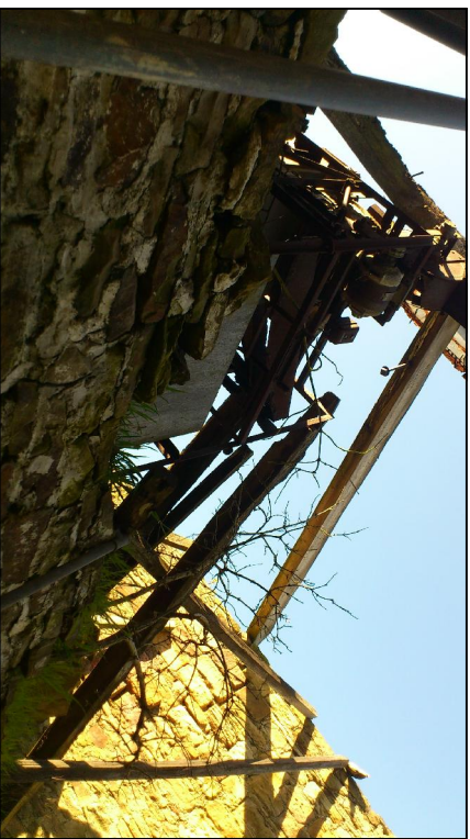
PICTURE L SHOWING REMAINS OF ROOF STRUCTURE
