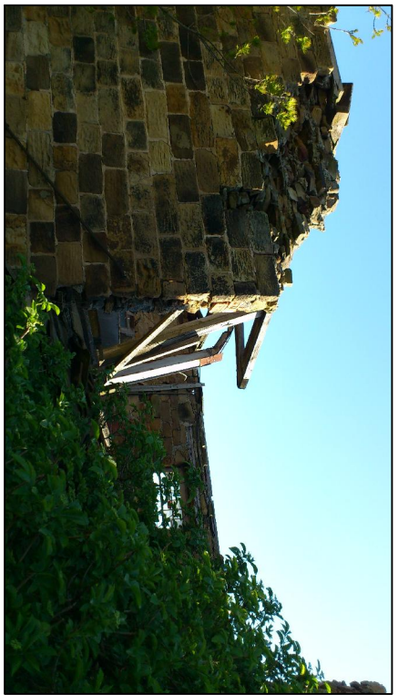
PICTURE R SHOWING MISSING SECTION OF EXTERNAL WALL
