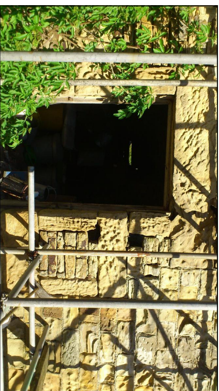
PICTURE I SHOWING WEATHERED SANDSTONE WALL AND DOORWAY
