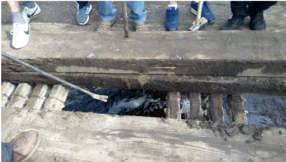
Above: Fig 1.5.5 View with x1 No. Timber Cross Beam removed – co positive connection between steel girder and Timber Cross Members – self weight and contact only.
