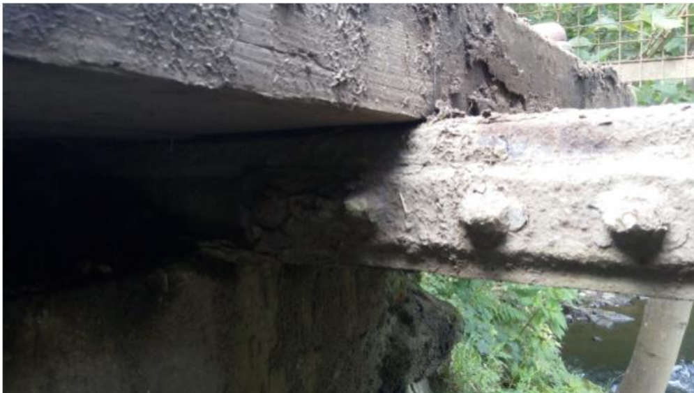
Above: Fig 1.5.6 View with x1 No. Timber Cross Beam removed – no positive connection between steel girder and Timber Cross Members – self weight and contact only – Note the fish plate connection
