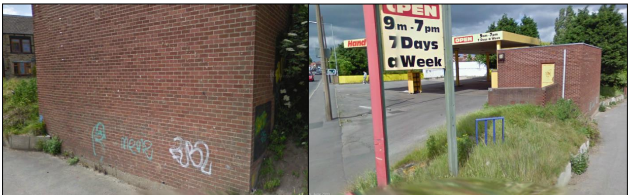
Evidence of graffiti
