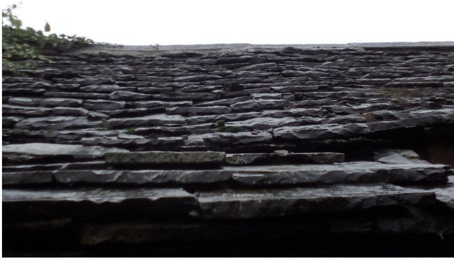
Image 7: Gaps between tiles on roof of B3
