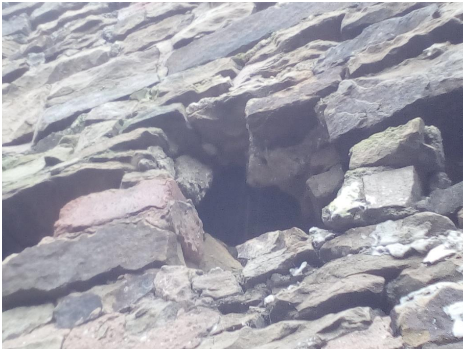
Image 6: Large crevice in north wall of B2
