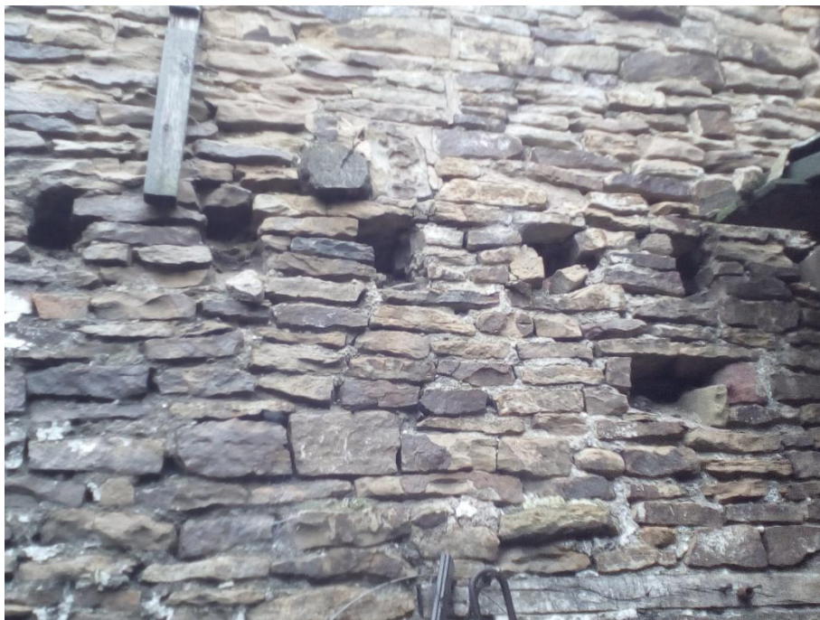
Image 4: B2 interior - holes within south wall
