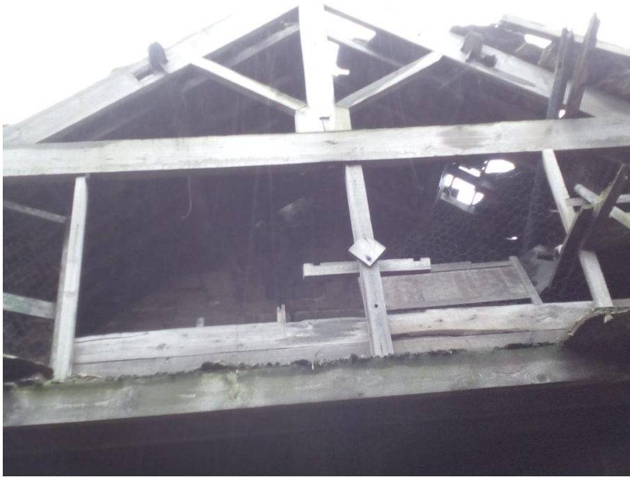
Image 5: B2 interior - showing collapsed roof and remaining first floor section
