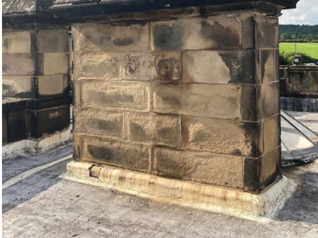
3.23 Example of flashing degradation to the base of the chimney stacks.
