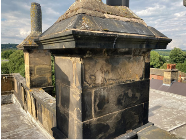
3.21 Chimney stack stonework in need of indent repair
