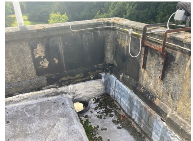
3.17 Moss build up in the roof gutters
