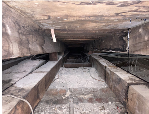
3.19 Evidence of water ingress damage on the roof rafters.
