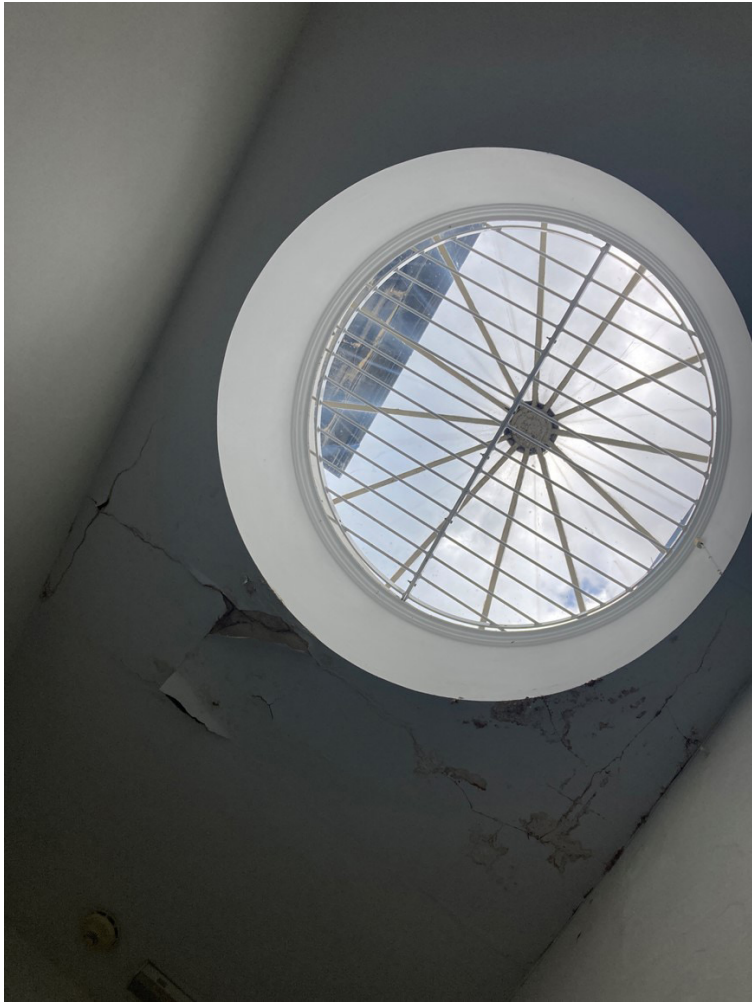
3.18 Internal plaster damage relating to water ingress around the roof lights.
