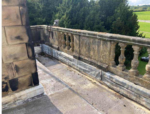
3.20 Degradation of the lead flashing around the balustrade
