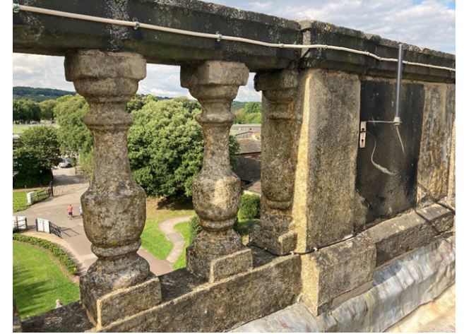
3.24 Weathering to the perimeter balustrading.
