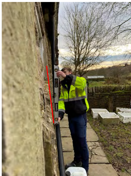
Figure 13: Front Elevation Wall Deviation
