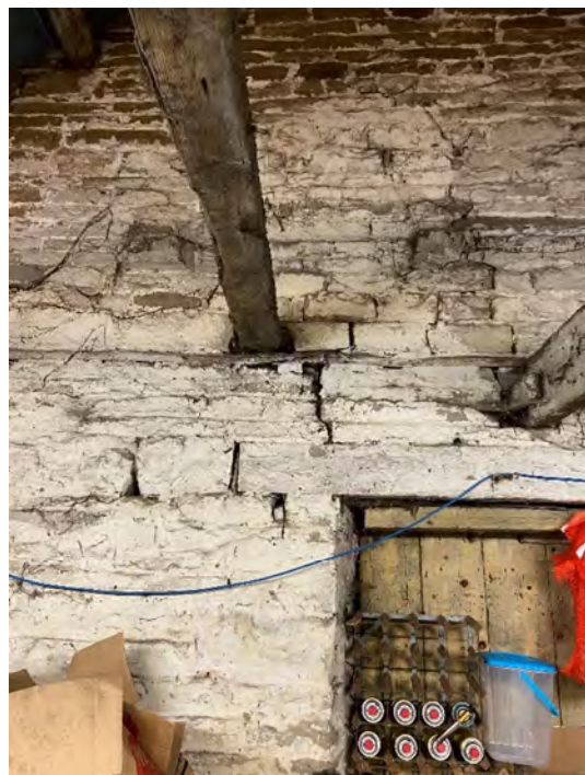
Figure 19: Workshop Internal Wall Cracks
