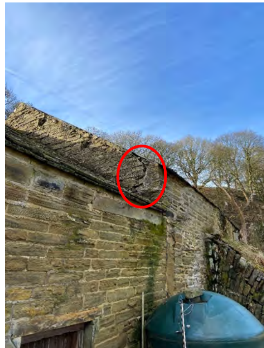
Figure 39: Barn Crack in Gable (Cracks Highlighted)
