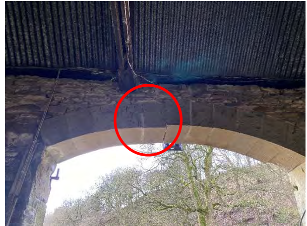
Figure 28: Barn Dropped Key Stone in Arch (Dropped Keystone Highlighted)
