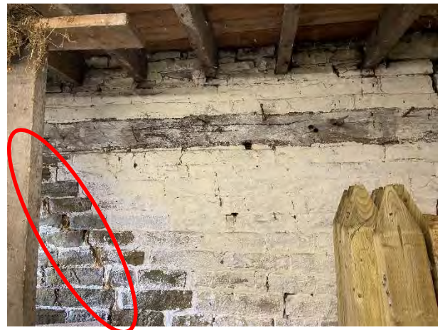
Figure 30: Barn Cracks in Dividing Wall (Cracks Highlighted)
