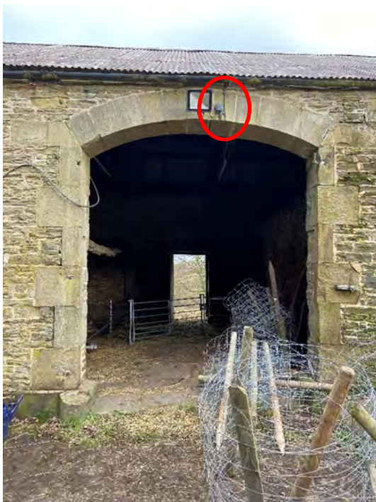
Figure 21: Barn Front Arch Entrance (Dropped Keystone Highlighted)
