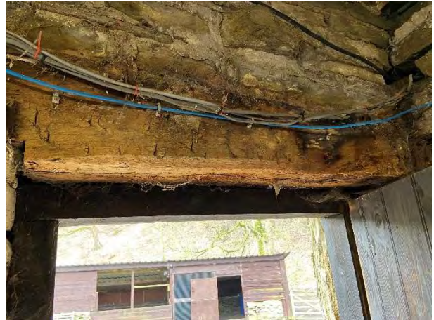
Figure 17: Workshop Rotten Door Lintel
