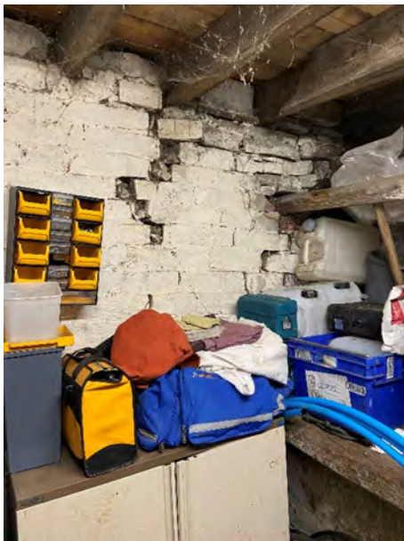
Figure 29: Barn Cracks in Dividing Wall
