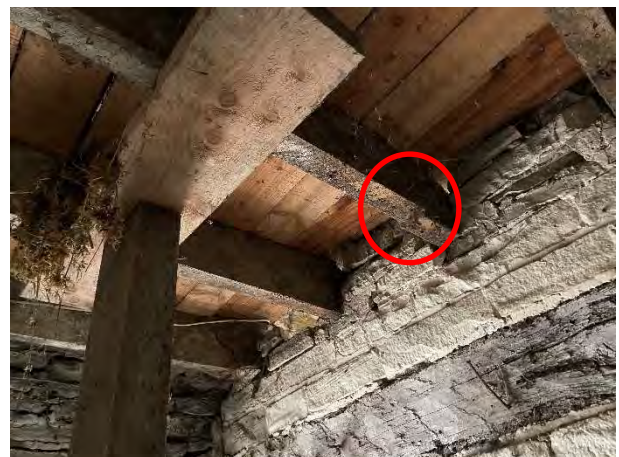
Figure 26: Propped Timber Joists with Split in Floor Joist (Cracked Joist Highlighted)
