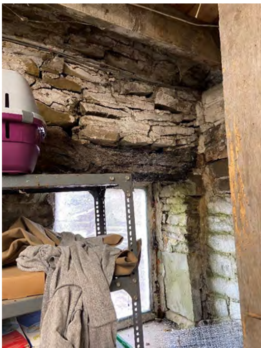
Figure 25: Barn Internal Rotten Lintel with Loose Masonry Above
