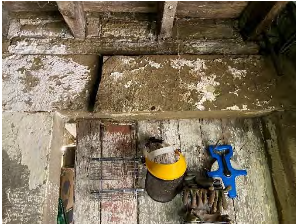
Figure 23: Barn Internal Cracked Lintel
