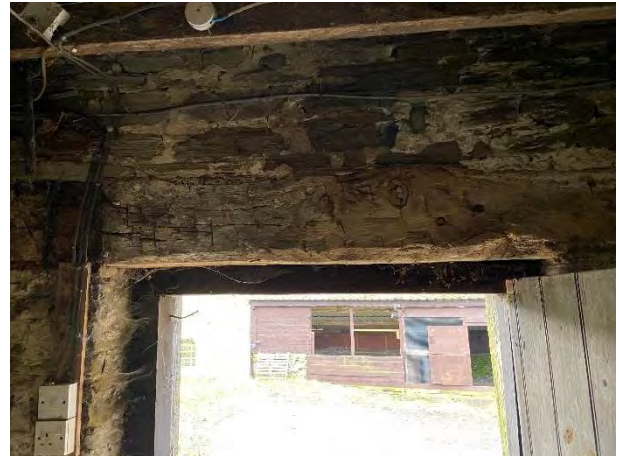
Figure 24: Barn Internal Rotten Timber Lintel
