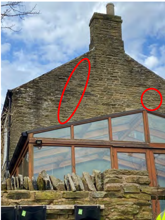
Figure 6: Farmhouse Side Elevation (Crack Locations Circled)
