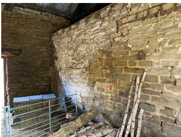
Figure 31: Barn Cracks in Dividing Wall
