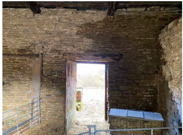
Figure 33: Barn Rotated Lintel Over Door
