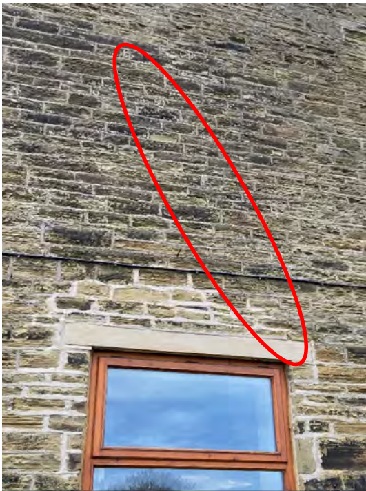
Figure 10: Farmhouse Rear Elevation Lintel (Crack Location Highlighted)
