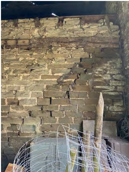
Figure 32: Barn Cracks in Dividing Wall
