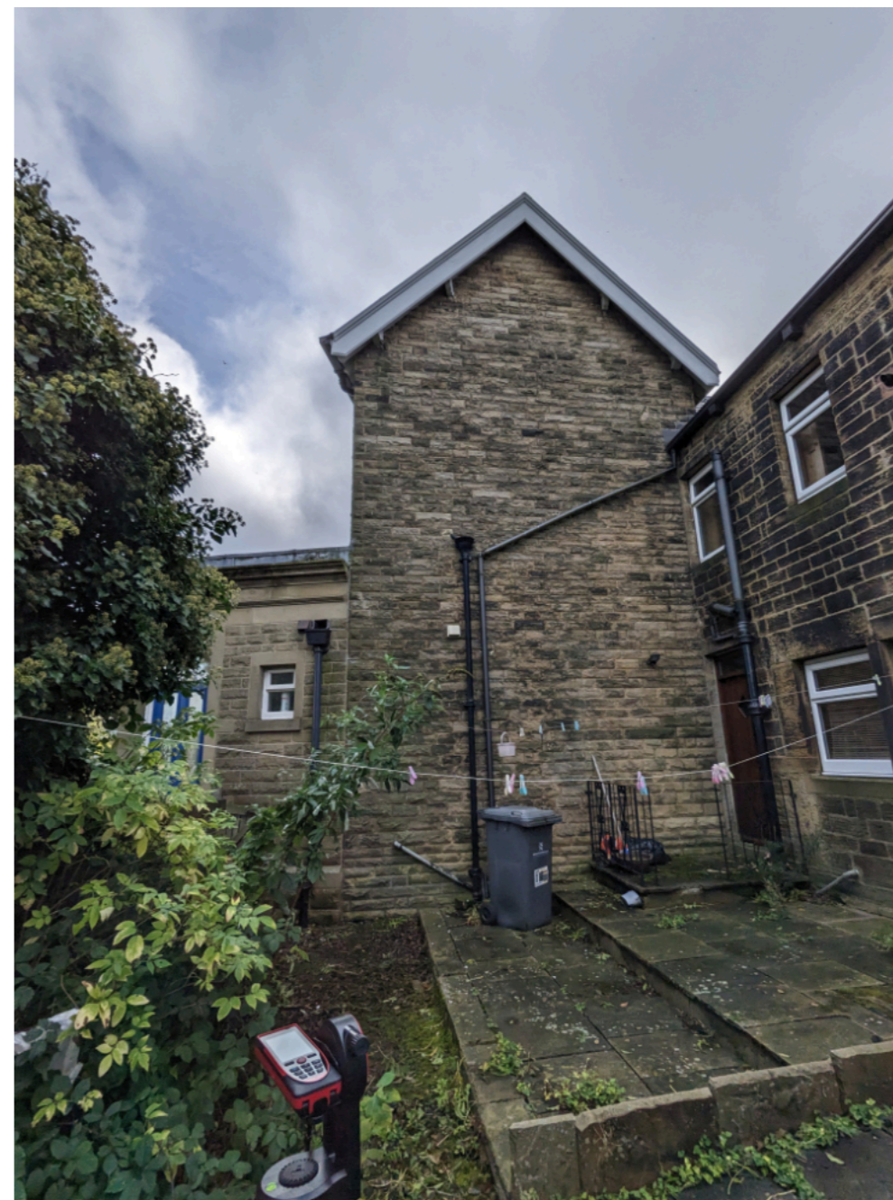
2306 - 103 High Street, Penistone Rear (North) elevation viewed from access route to rear of No.101 High Street yard
