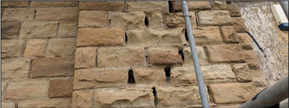
Plate 8. Open joints in wall and gaps between window boards and masonry
