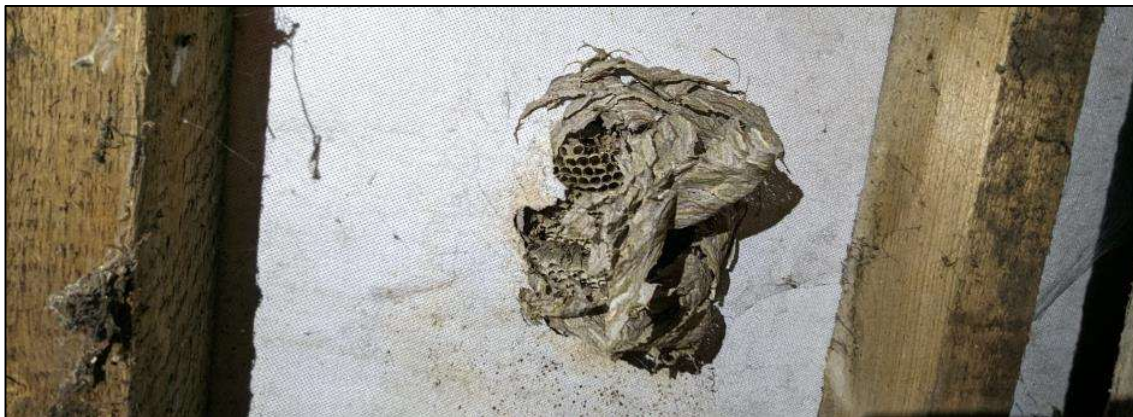
Plate A2.2. Damage to a breathable roofing membrane adjacent to a wasp nest
