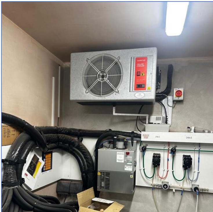
Figure 4.3: Internal Beer Cellar Plant
