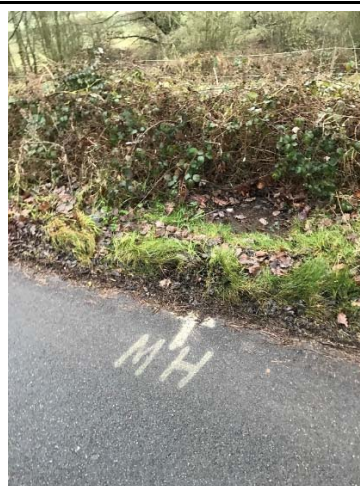
Combined manhole (in Cote Lane)
